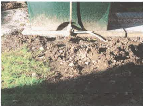
Oil tank and pipework February 2017
