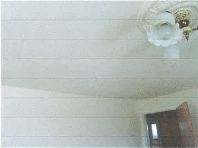
Living room ceiling February 2017
