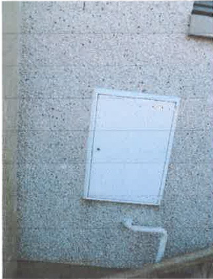
External meter cupboard February 2017
