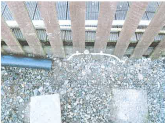
Oil supply pipework February 2017
