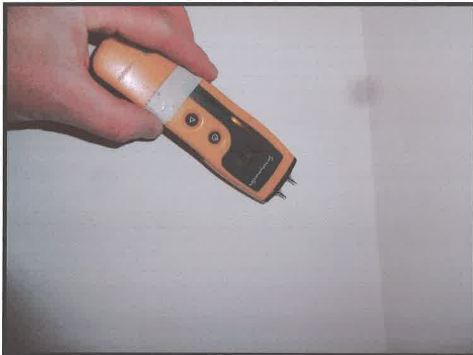
Figure 6 Bedroom - Meter reading (18%) front corner wall, mid height.
