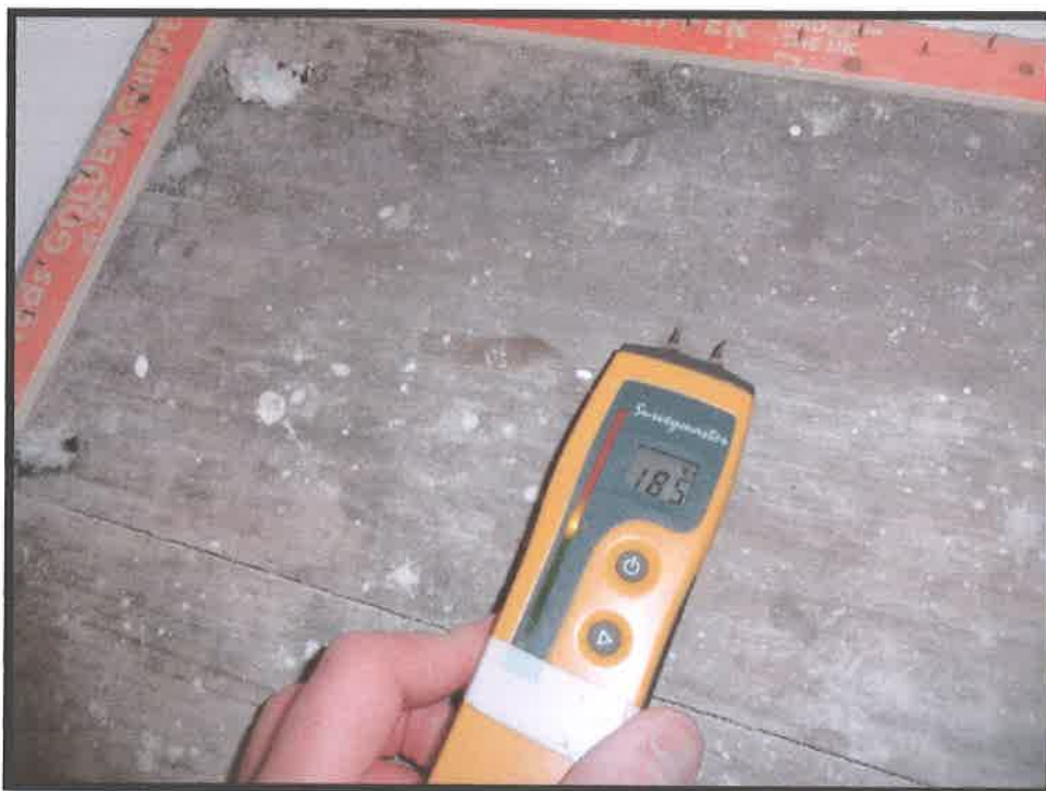
Figure 7 Bedroom - Meter reading (18%) at top surface of flooring.
