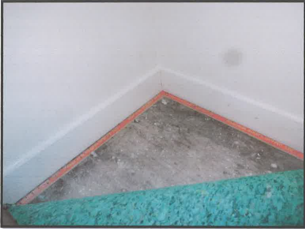
Figure 4 Bedroom - surface of flooring in front corner of room
