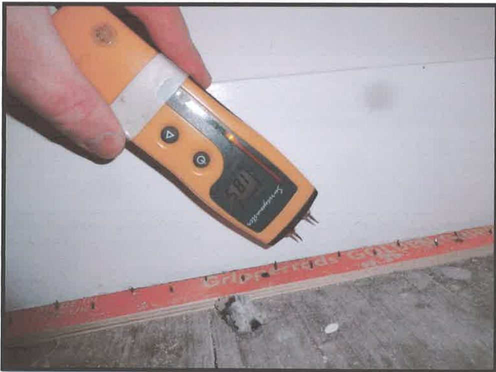
Figure 5 Bedroom - Meter reading (18%) at skirting board.
