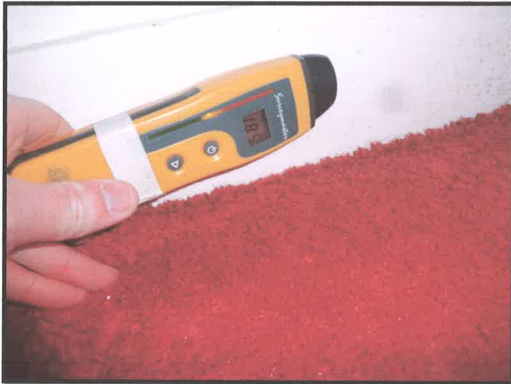
Figure 8 Bedroom wardrobe - Meter reading (18%) and residue of mould growth to skirting
