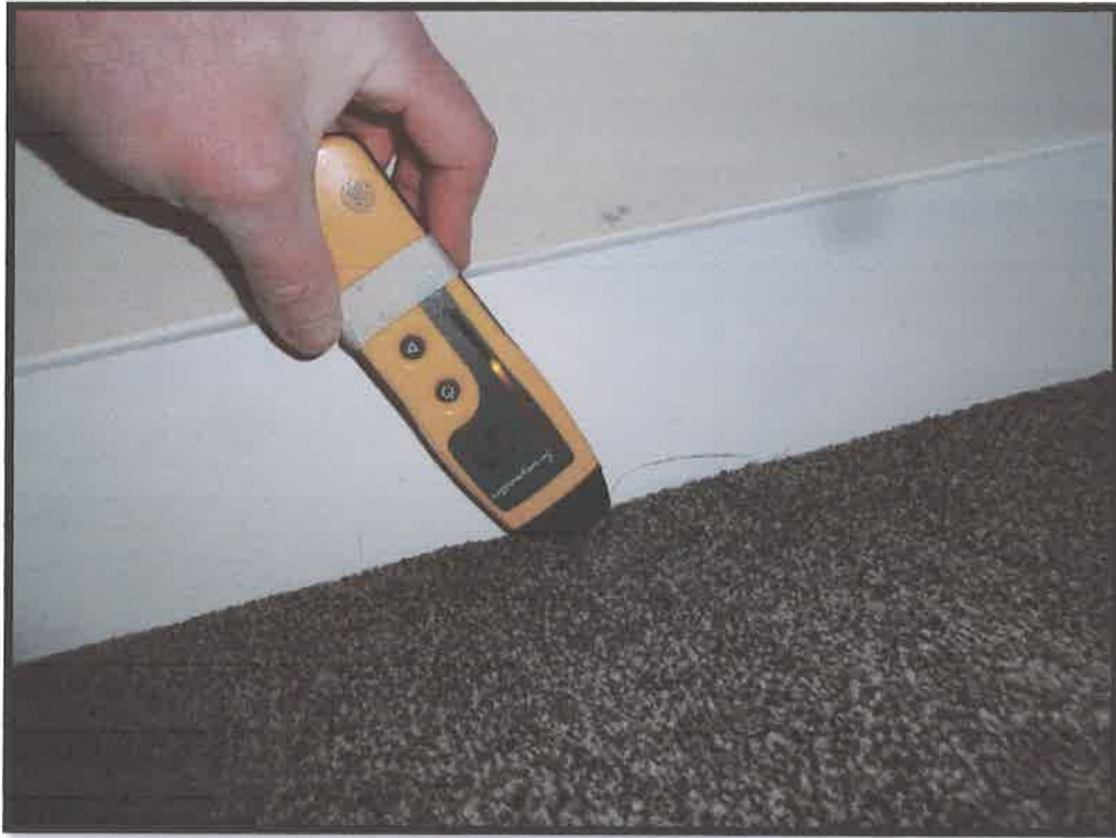
Figure 10 Lounge - Meter reading (18%) skirting below front window, mould residue above skirting
