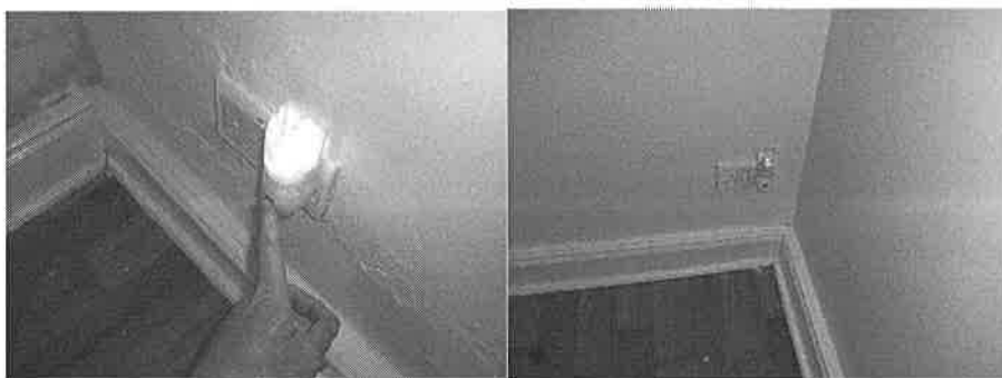
Electrical Sockets May 2016
