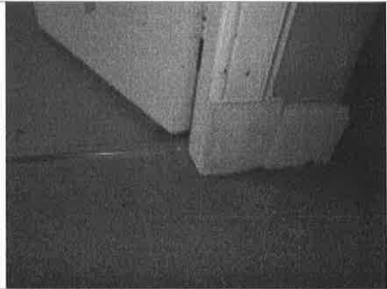
Plinth block to base of bedroom door frame
