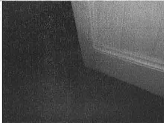
Carpet in main bedroom secured at skirting
