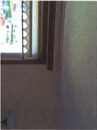
Redecorated area above curtain rail
