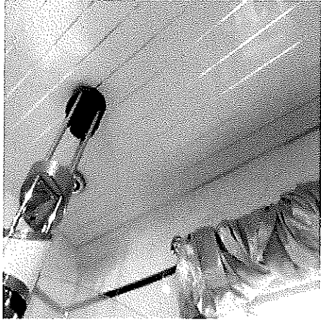
Bathroom Ceiling 15 th April 2015
