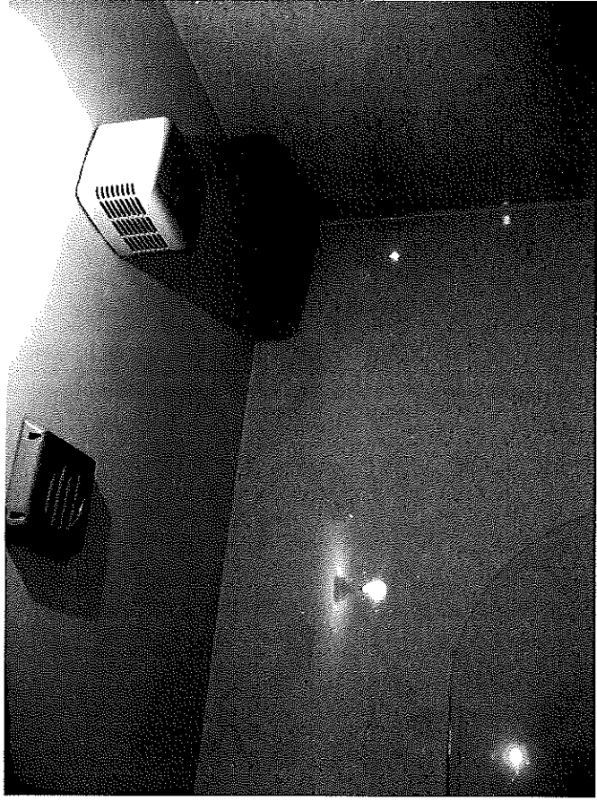
06 - Bathroom - extractor now working
