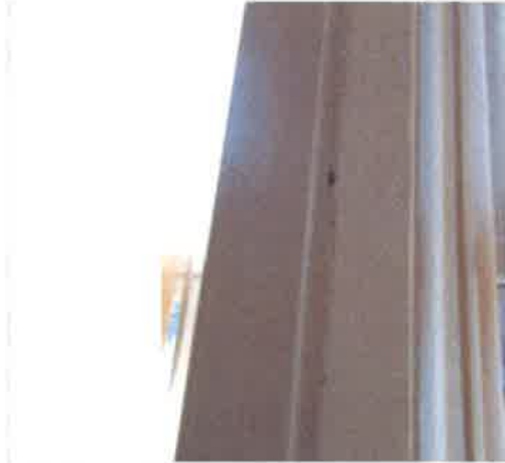
Living Room windows - slight damage to adjoining paintwork
