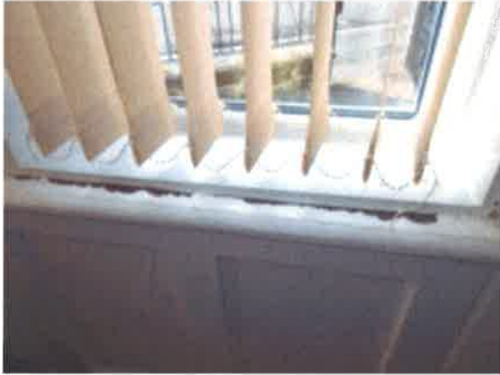
Living Room windows - slight damage to adjoining paintwork
