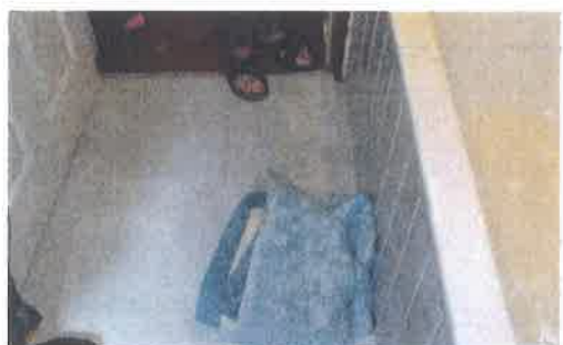
Photo 7 – Dampness in floor
