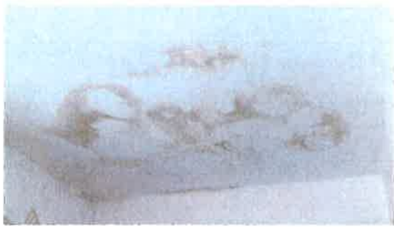
Photo 2 – Damp Living room ceiling
