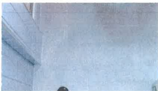
Photo 6 – Dampness in floor
