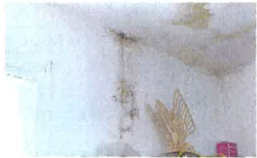
Photo 3 – Water damaged L/R wall
