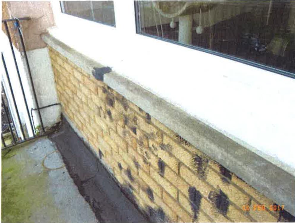
Open joints in brickwork below Lounge window
