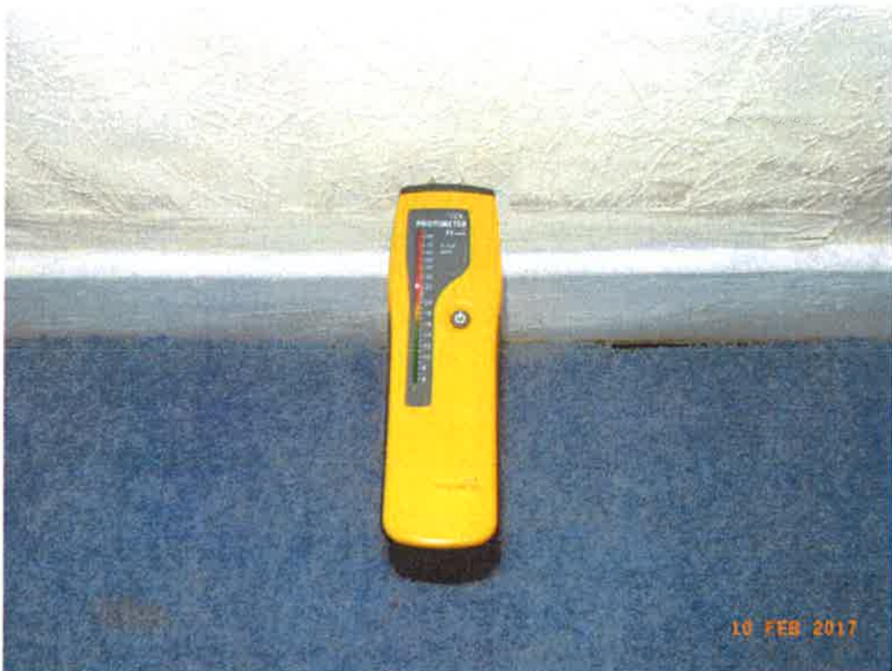
High damp meter reading in Lounge
