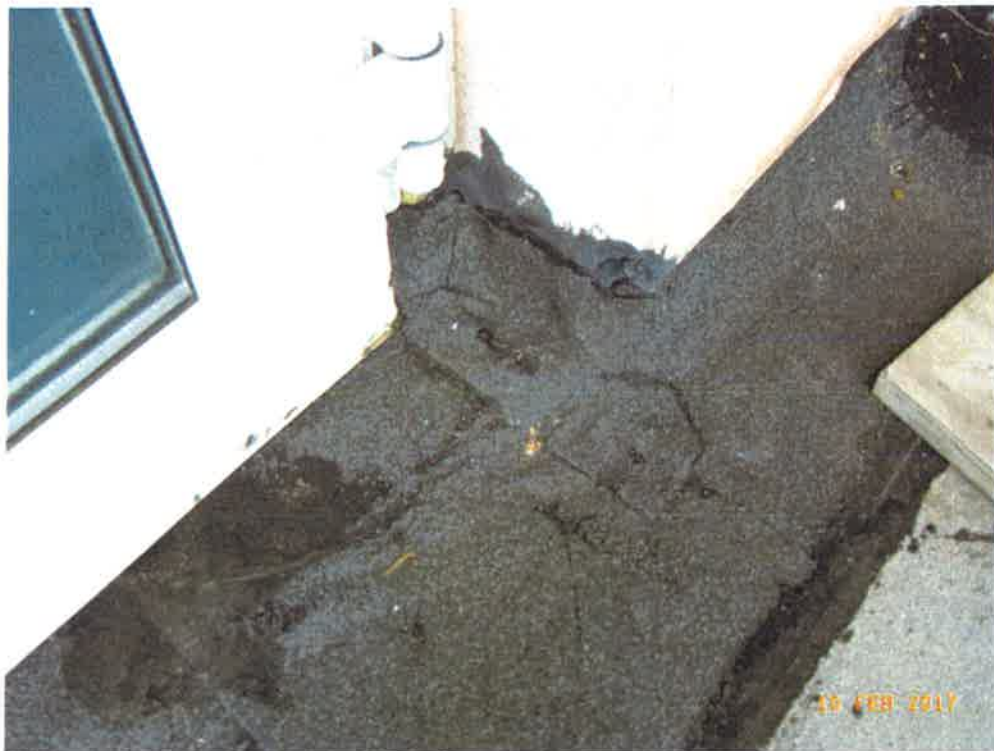
Lounge door – flashing at threshold
