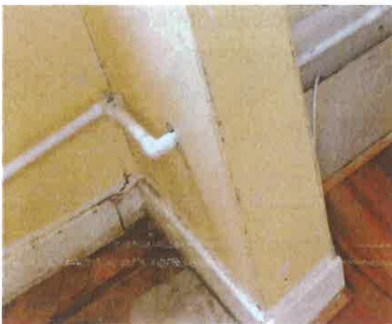
(10) Damaged floor covering rear bedroom
