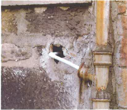
(6) Hole in wall at condensate pipe
