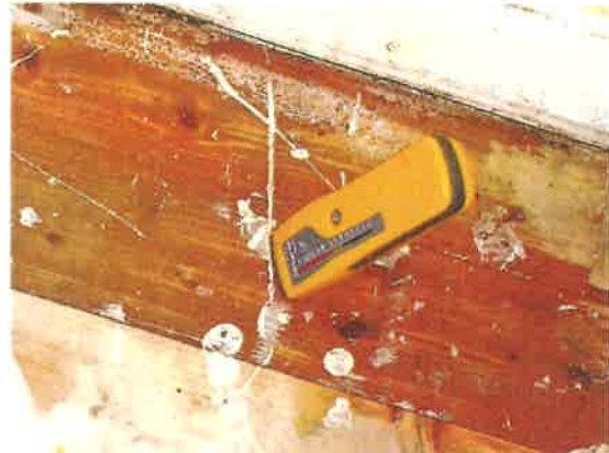
(9) Saturated floor below condensate pipe
