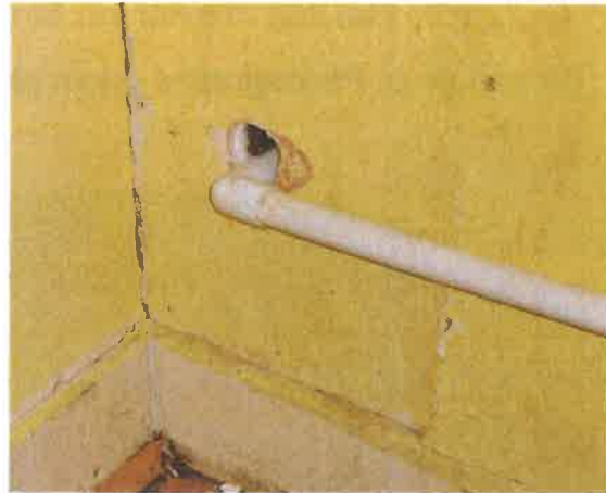
(7) Hole in rear bedroom wall at pipe
