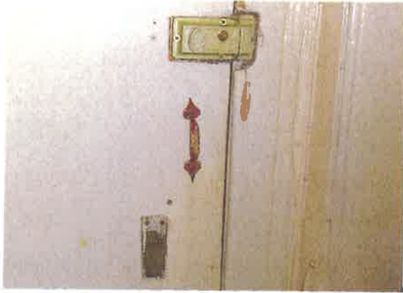
(12) Replacement "Yale" lock
