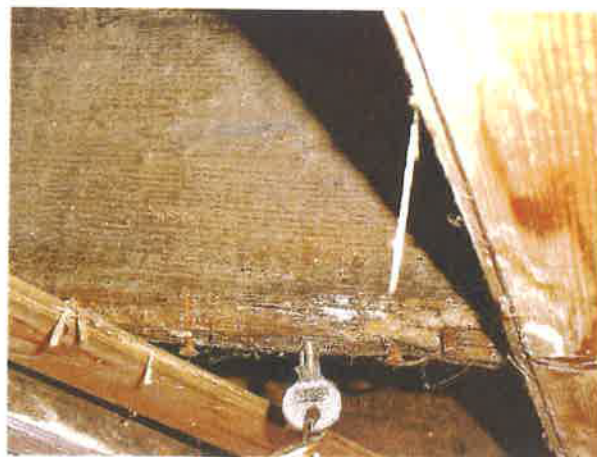
(5) Rot in joist below bath
