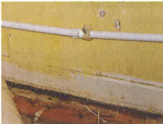
(8) Broken joint in condensate pipe
