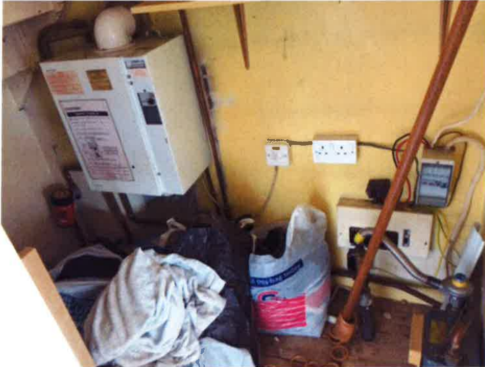
Gas boiler and electrical installation
