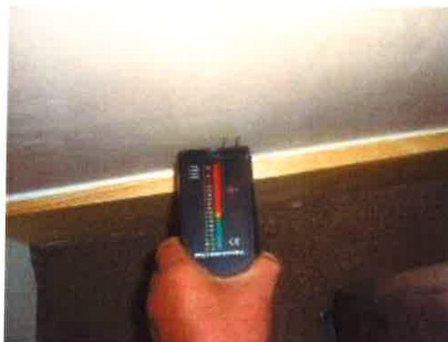
The re-plastered walls in the kitchen and lounge remain to be decorated.
