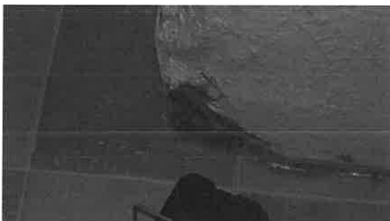
Photo 4 – Silicon filled hole in kitchen
