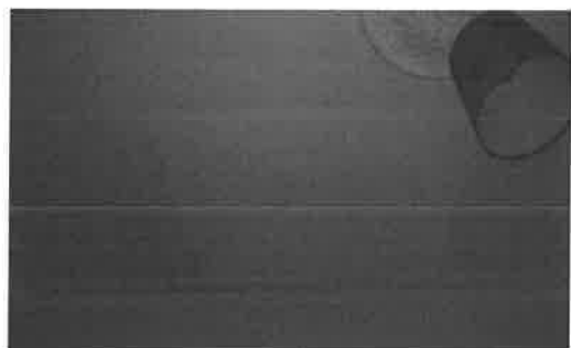
Photo 5 – Crude patch repair in L/Room
