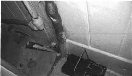
Photo 2 – Rodent access point in bathroom
