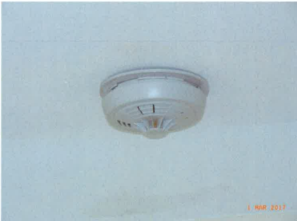
Kitchen heat alarm
