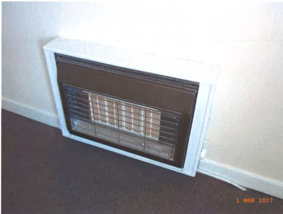
Living room gas fire
