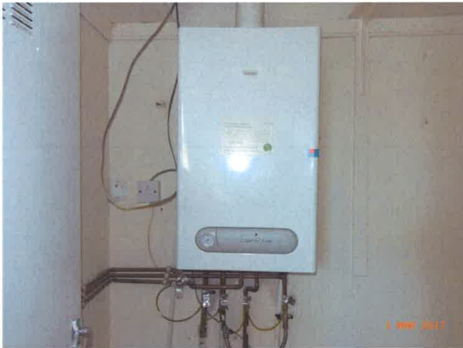
Central heating boiler
