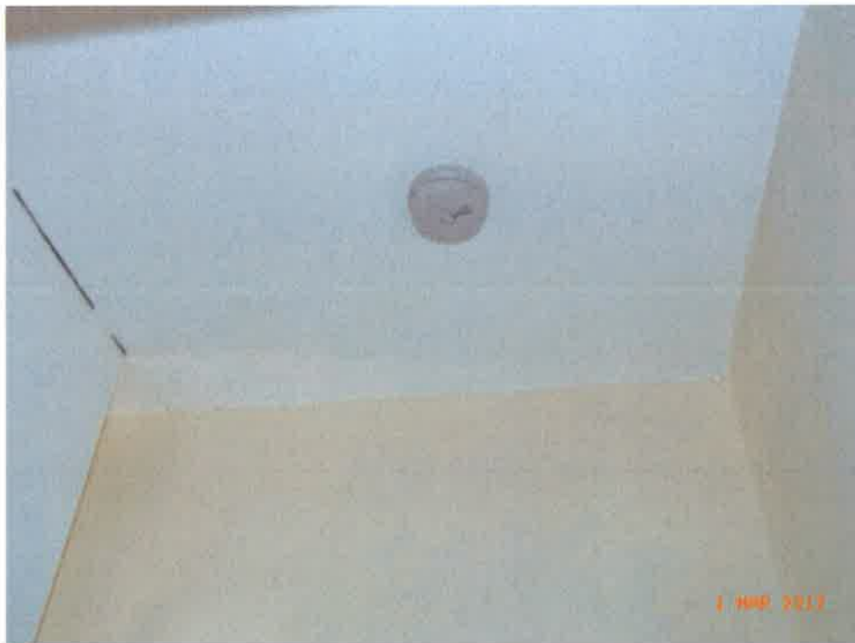
Hall smoke detector
