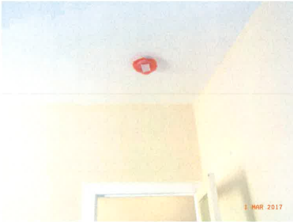
Living room smoke detector
