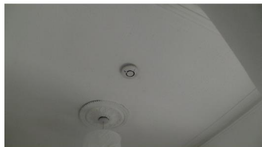
Photo 5 – Smoke alarm in Hallway
