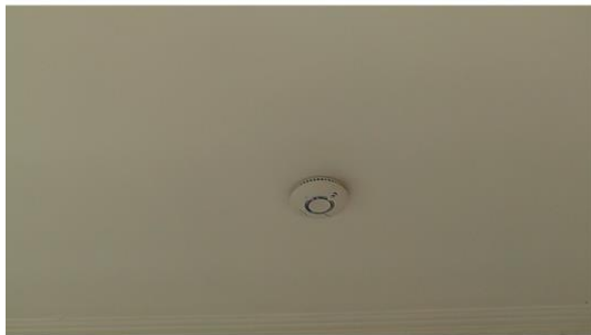
Photo 4 – Smoke alarm in Living Room
