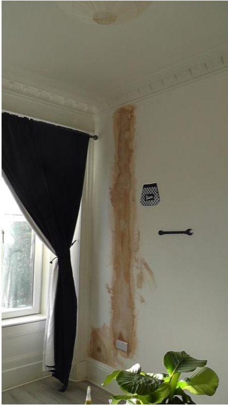
Photo 2 – Dry walls and ceiling in Living Room
