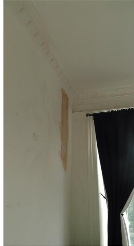
Photo 3 – Dry walls and ceiling in L/Room
