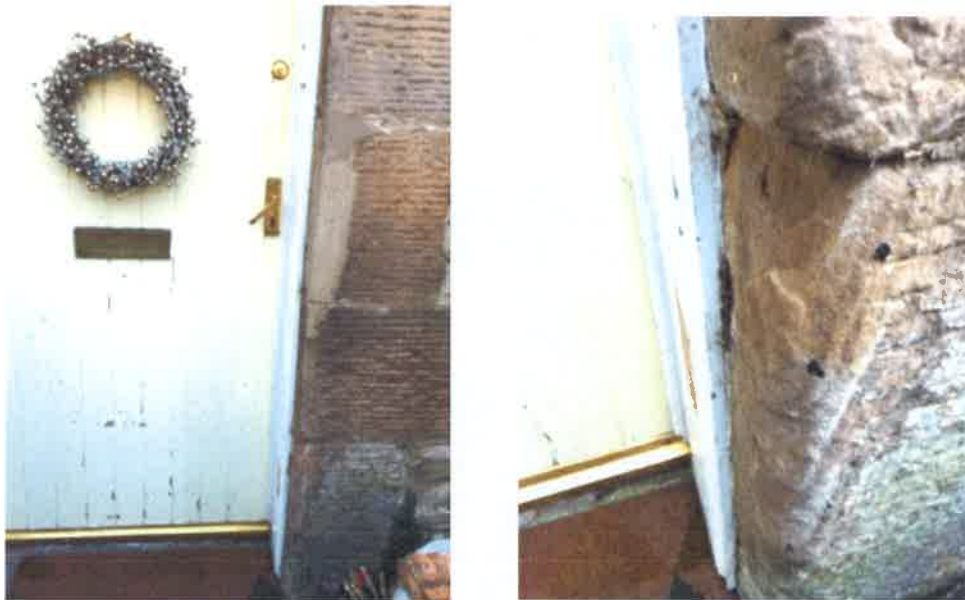
Front door and close up of wall to right hand side of front door showing gaps in pointing around door frame and external wall
