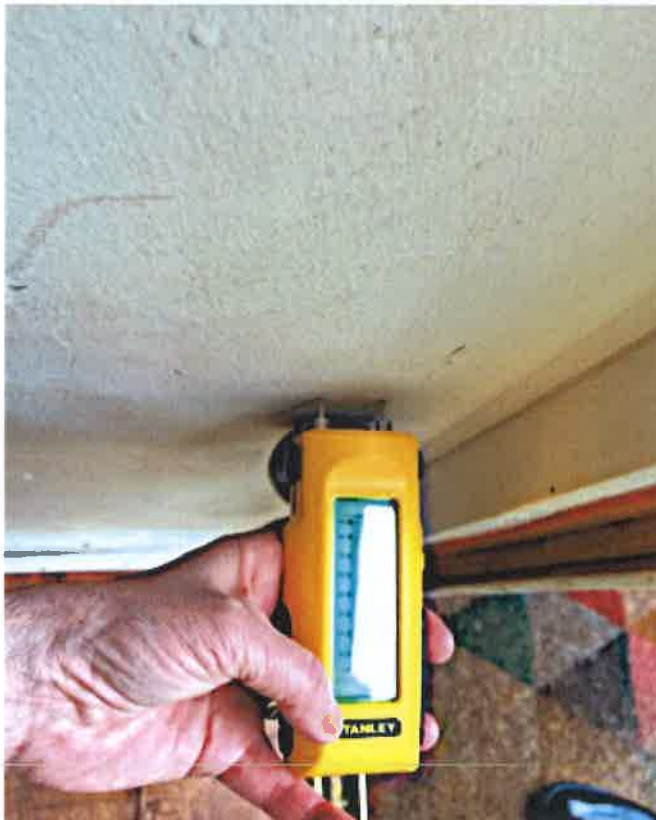
Damp meter reading taken on the left internal wall adjacent to the front entrance door
