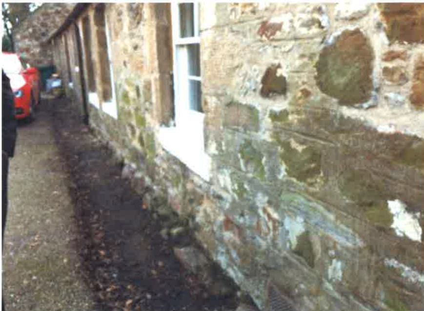
Channel dug along front elevation in front of hall cupboard and living room to the left hand side of front entrance door
