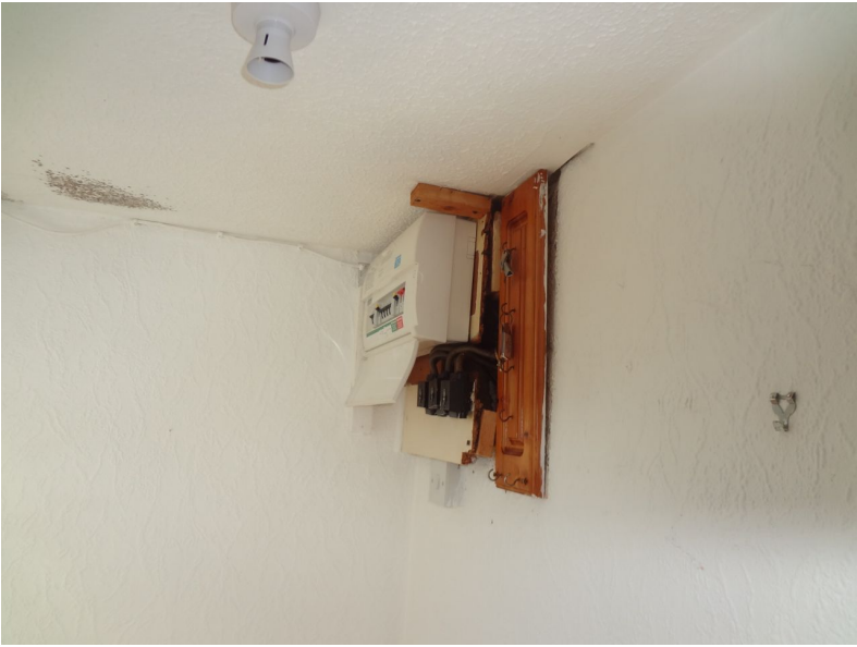
Electrical Distribution Board
