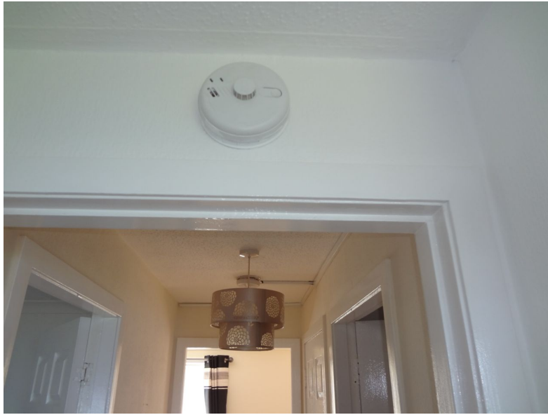
Interlinked Heat Detector in Kitchen
