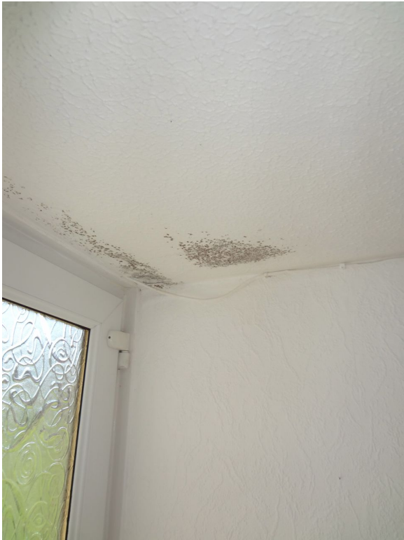
Mould on ceiling at Front Door
