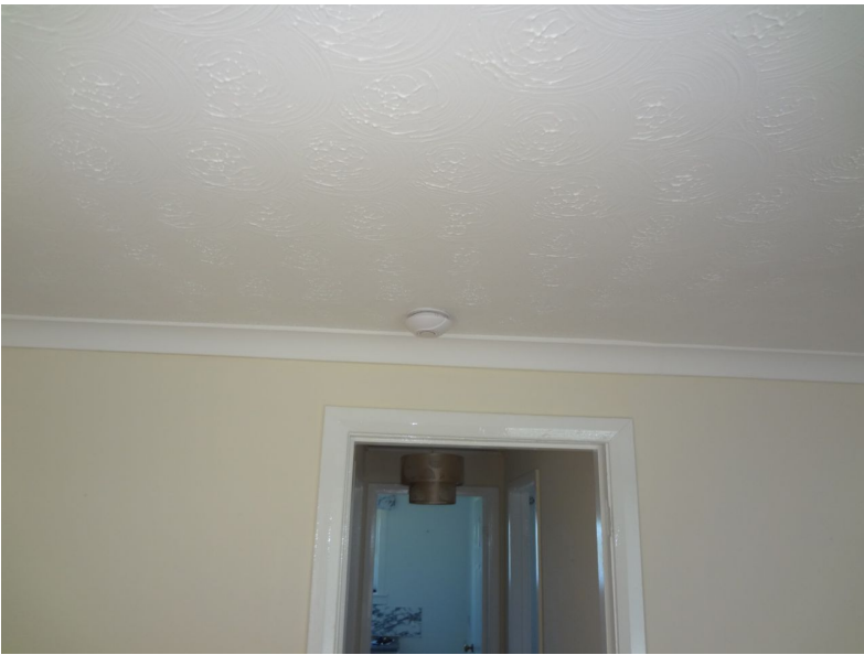
Interlinked Smoke Alarm – Living Room
