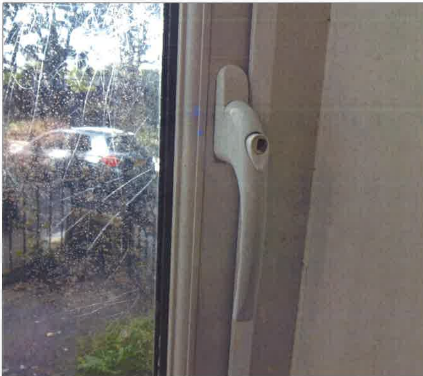
All windows tested, have a key and are able to open, close and lock
