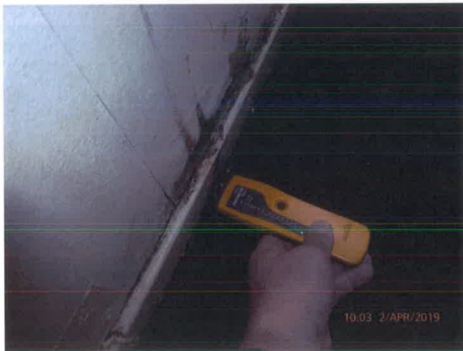
Damp meter reading below the window
