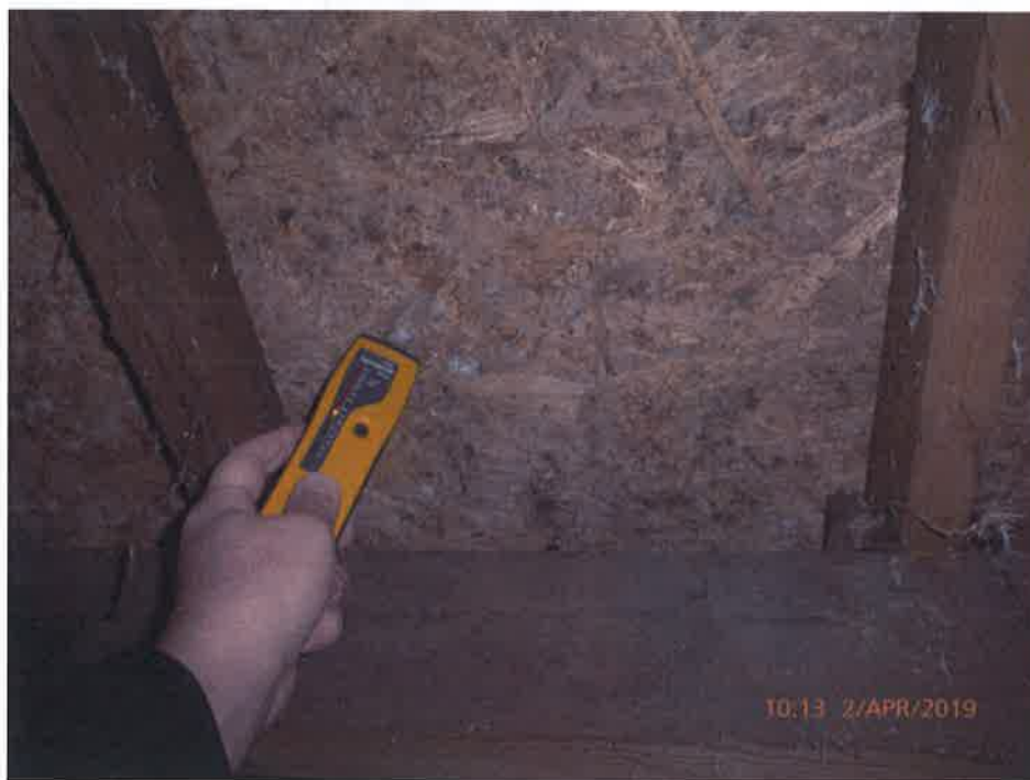
Meter reading in the roof space
