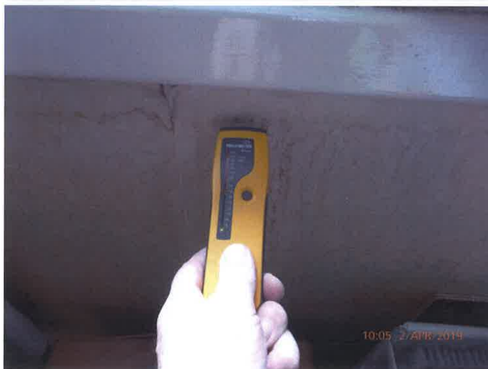
Staining below rear bedroom window
