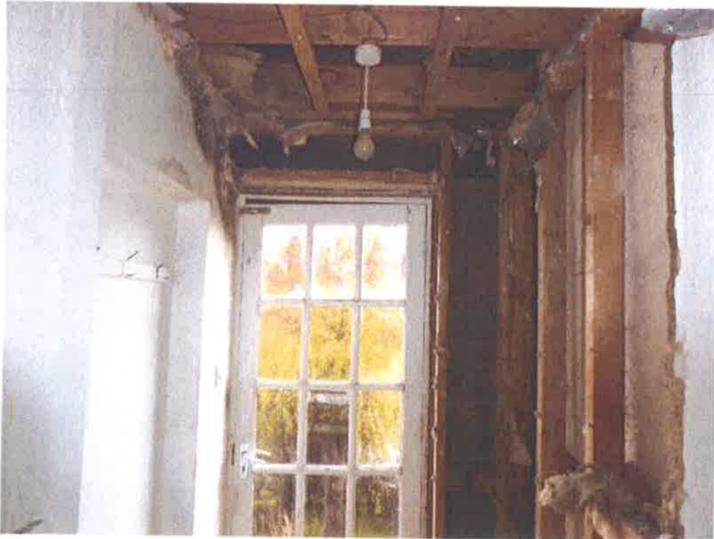
External rear door from kitchen corridor – unchanged but ceiling and wall stripped back and showing damp ingress
