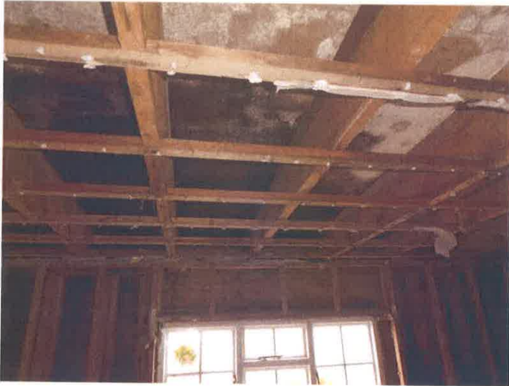
Flat roof and part external wall above middle bedroom showing water ingress to whole roof.
