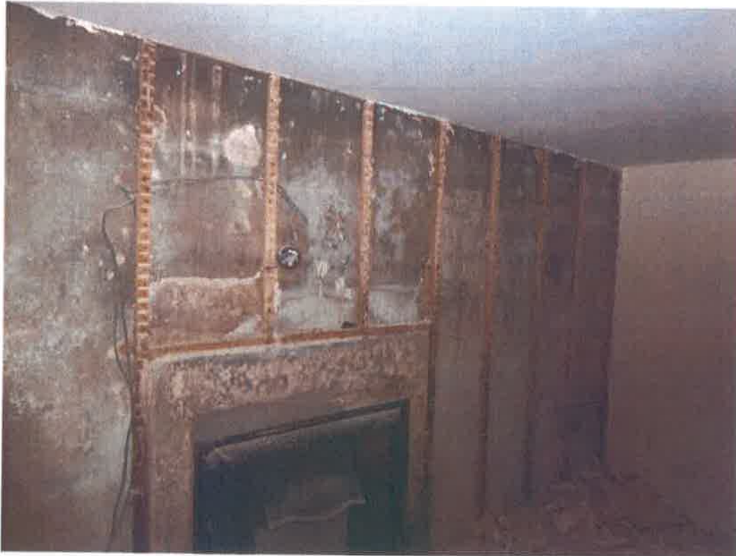
Ground floor bedroom gable wall stripped. Damp from chimney above not repaired.
