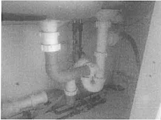
7 Plumbing to kitchen.
