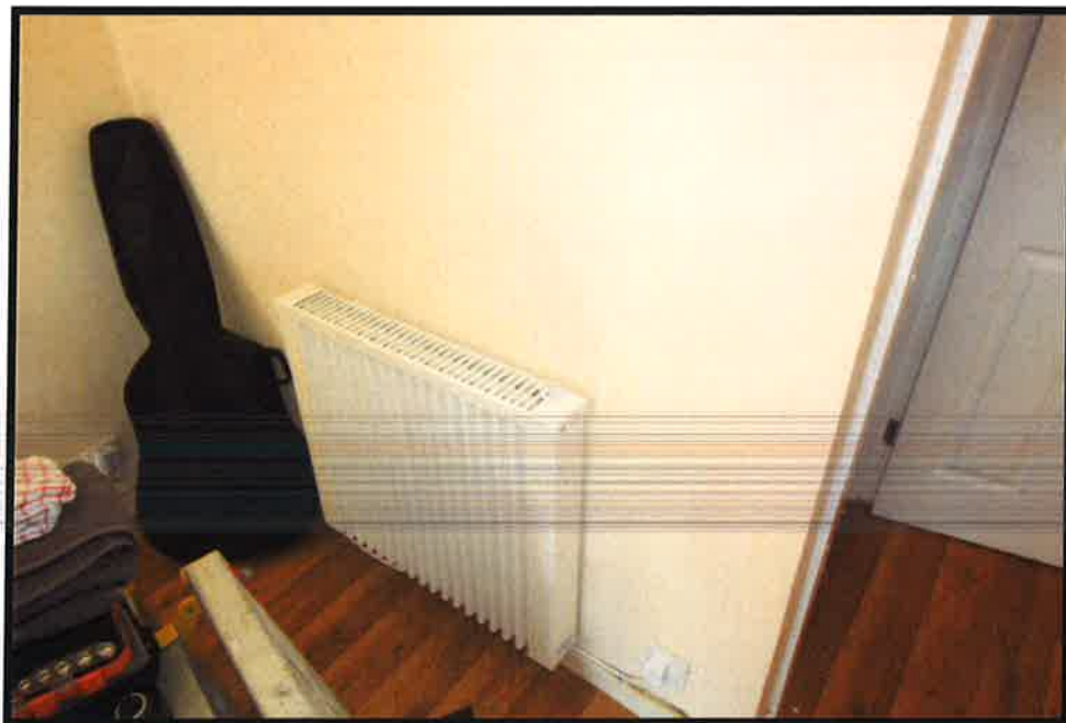
Photograph 3 Lounge - New heater.
