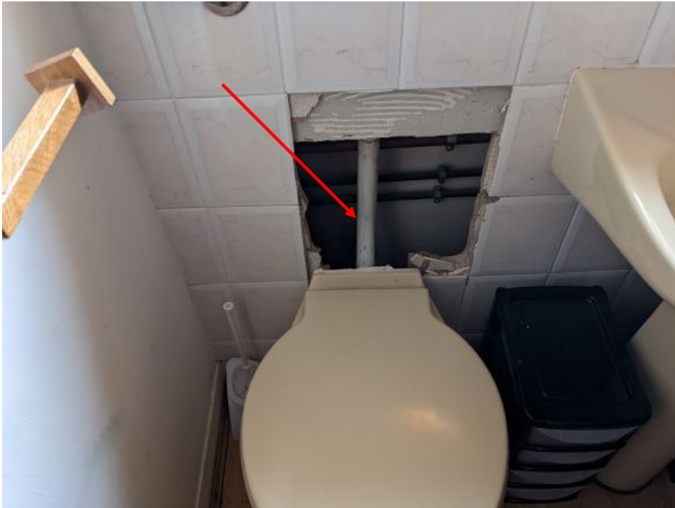
2 Hole behind bathroom WC
