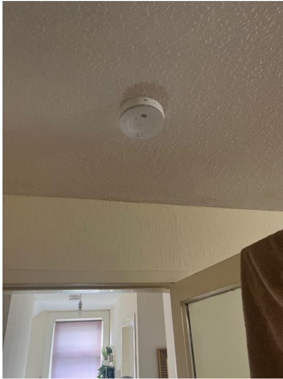
Photograph 2: Living room: smoke detector
