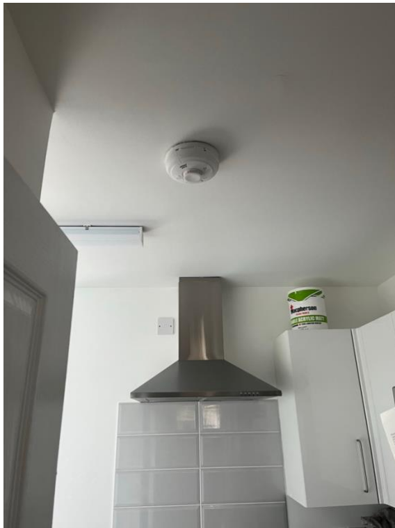
Photograph 3: Kitchen: heat detector
