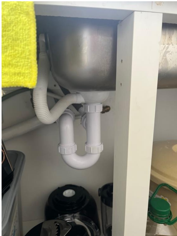
Photograph 5: Kitchen: under sink waste
