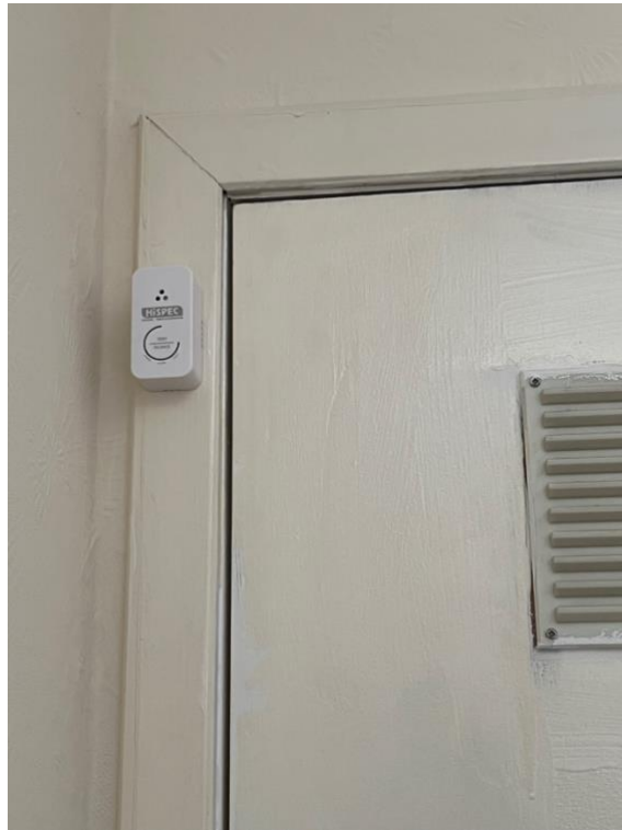
Photograph 13: Bedroom 2: Boiler cupboard; carbon monoxide detector
