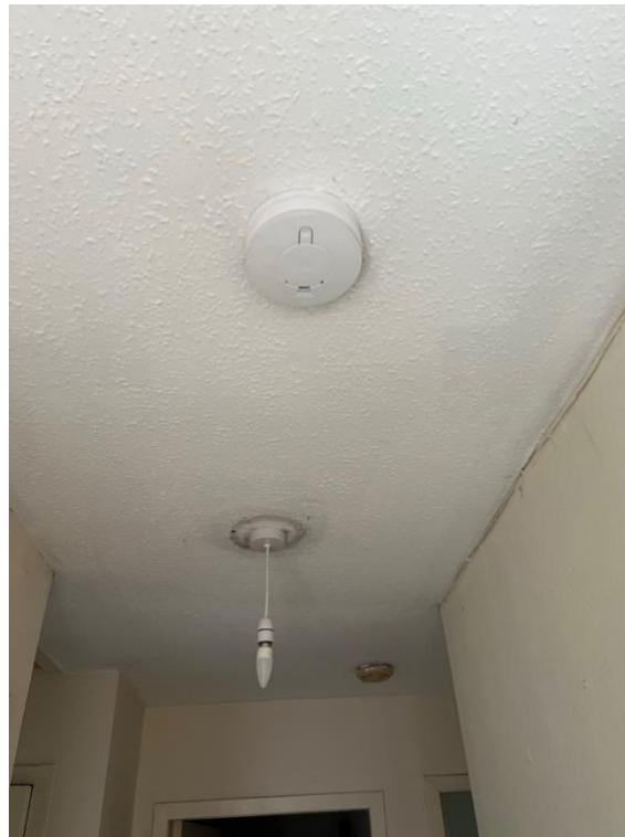
Photograph 1: Hallway: smoke detector
