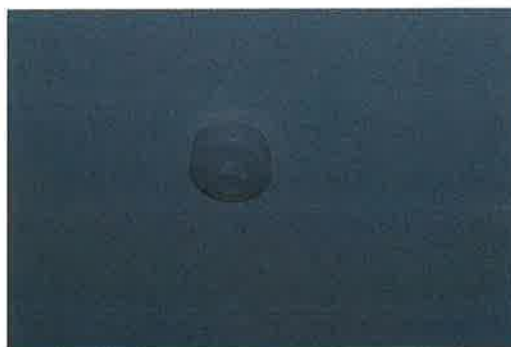
Photo 5 – Heat alarm in Kitchen
