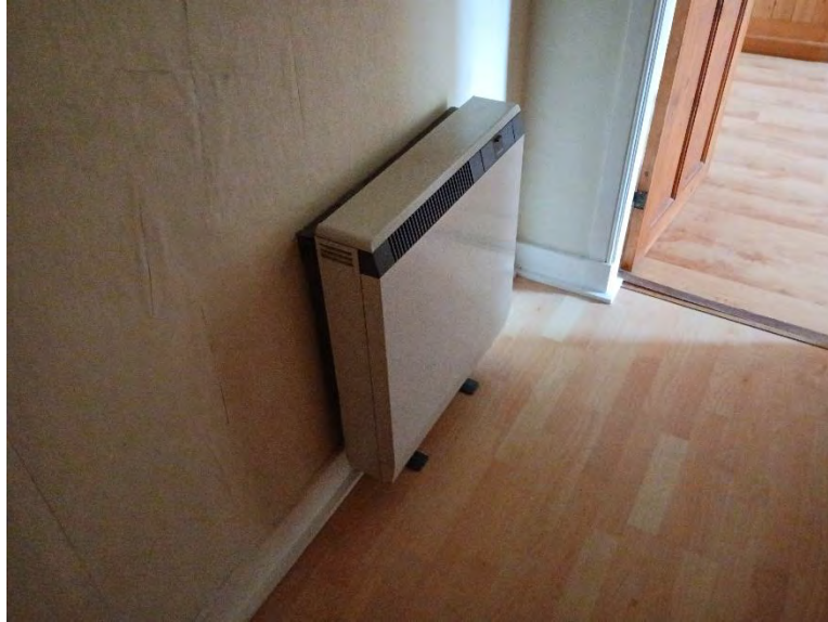
6 Aged electric storage heater in hall
