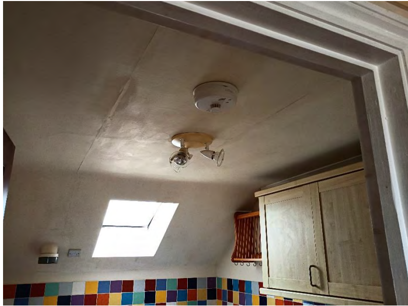
2 Heat detector in kitchen
