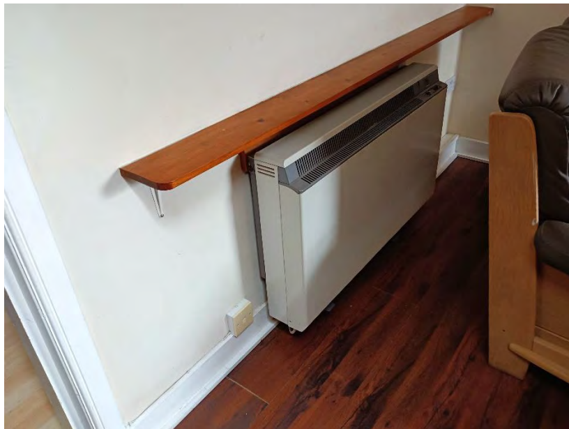
3 Aged electric storage heater in living room
