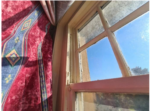
8 Defective sash cords to Bedroom sash and casement window.
