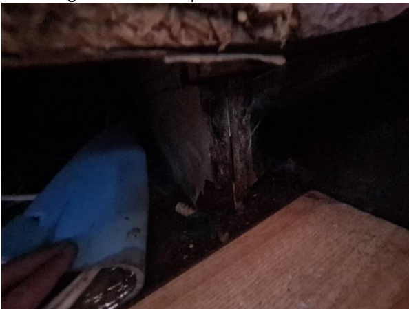
23 Area of timber decay below sink.
