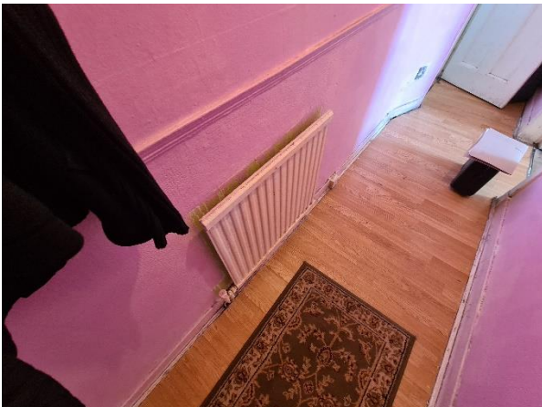
11 Redundant pressed panel radiator.
