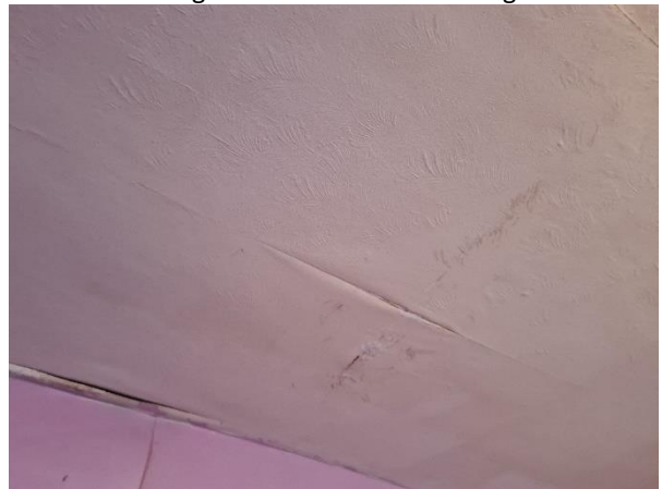
24 Loose ceiling paper and minor water staining to ceiling of Lounge.
