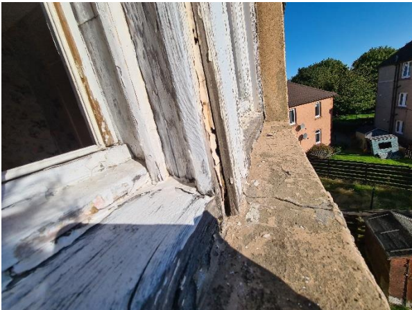
9 Poor condition of external timberwork at Bedroom window.
