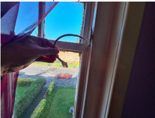
5 Snapped sash cord to Lounge window.
