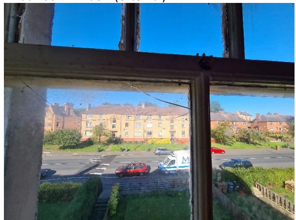
6 Cracked glass to Lounge window.
