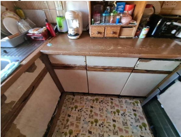
21 Damaged kitchen components.
