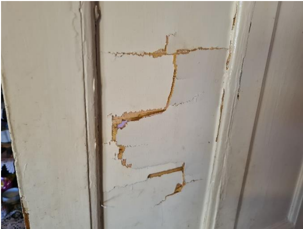
25 Lounge – damage to door.
