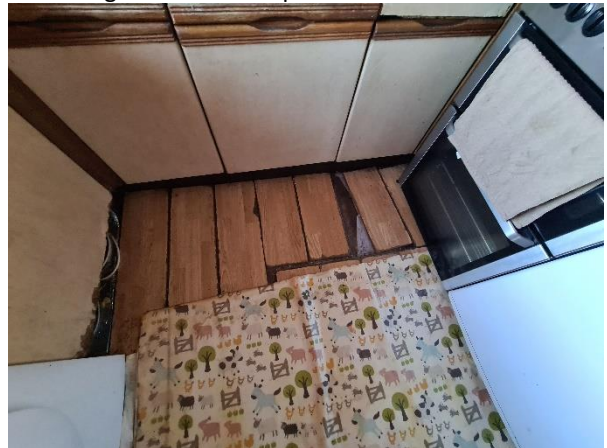
22 Water damaged laminate floor covering in Kitchen.
