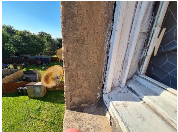
10 Defective perimeter seals to sash and casement window.
