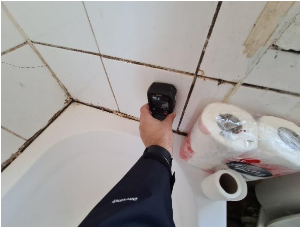
19 High moisture meter readings within Bathroom.
