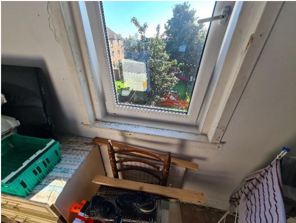
7 Replacement UPVC window to Bedroom.
