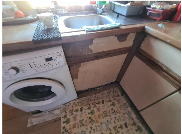
20 Damaged kitchen components.
