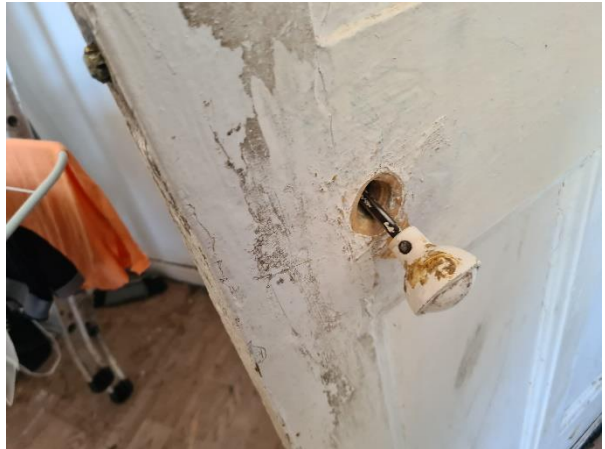
16 Loose door handle to Bedroom.
