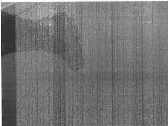
11 Bedroom – moisture check.
