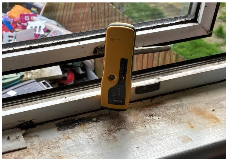
15. "Amber" damp reading at condensation stain rear bedroom
