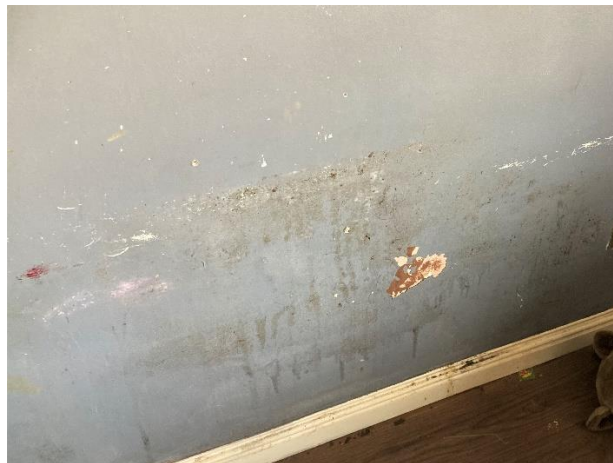
25. "Spillage staining" (DRY) in mutual living room/external pend wall
