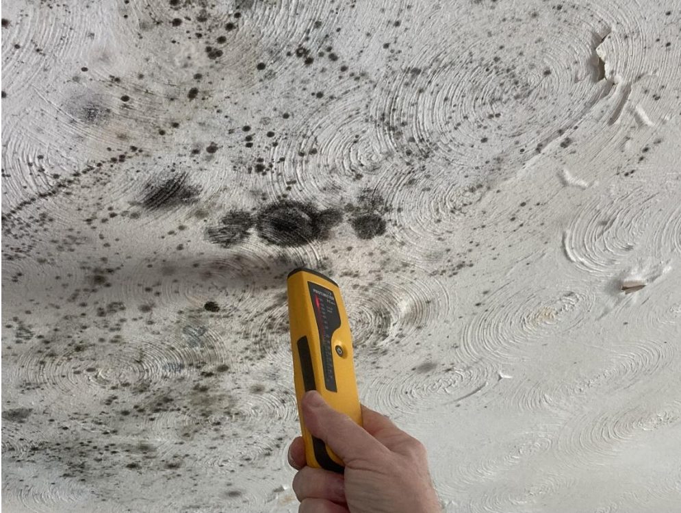
26. High damp readings in kitchen ceiling below bathroom
