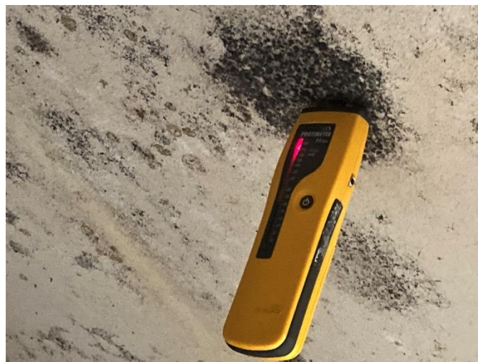
9. Damp "ceiling plaster" in attic
