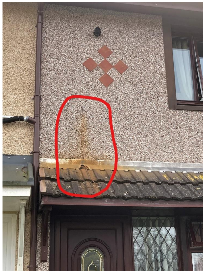
29 Residual staining below overflow pipe from boiler
