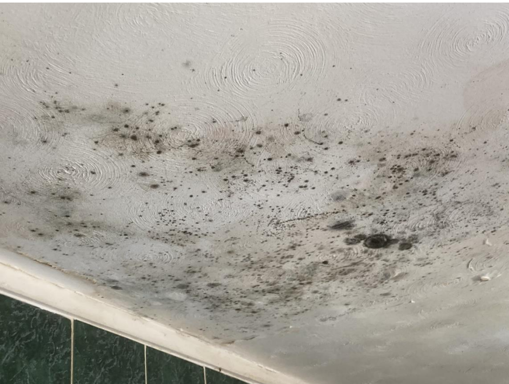
27. Damp staining kitchen ceiling below bathroom
