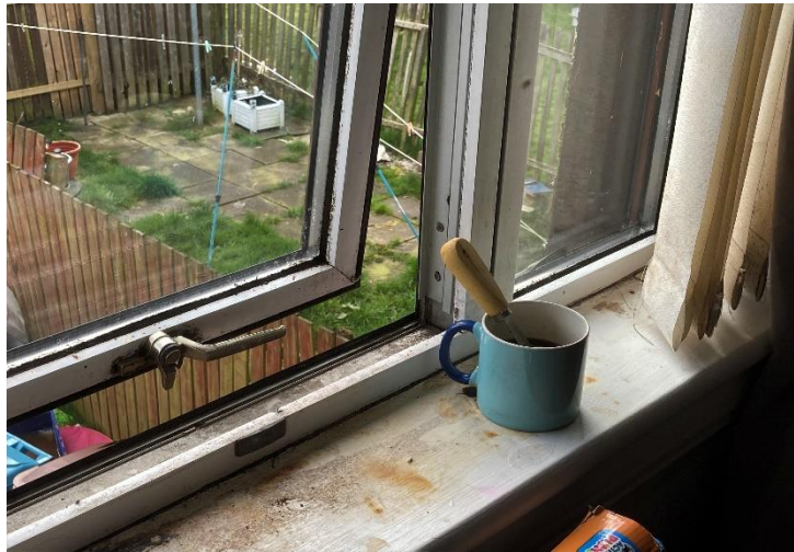
14. Condensation at rear bedroom window
