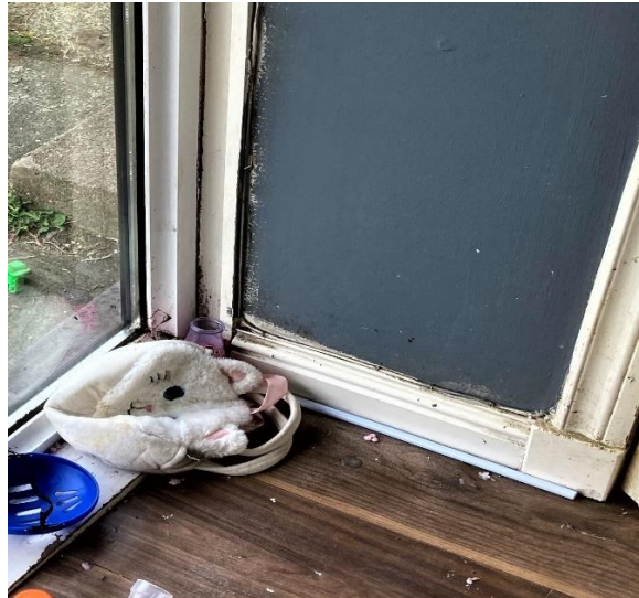
24 Condensation at skirting board and base of livingroom window
