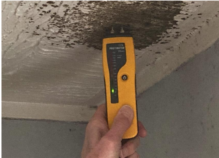
10. Staining (dry) front bedroom ceiling
