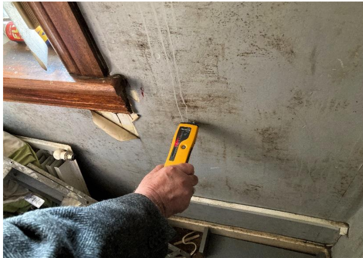
11. Damp wall plaster front bedroom
