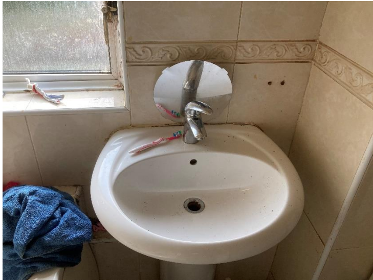
19. Condensation around wash hand basin and bathroom window
