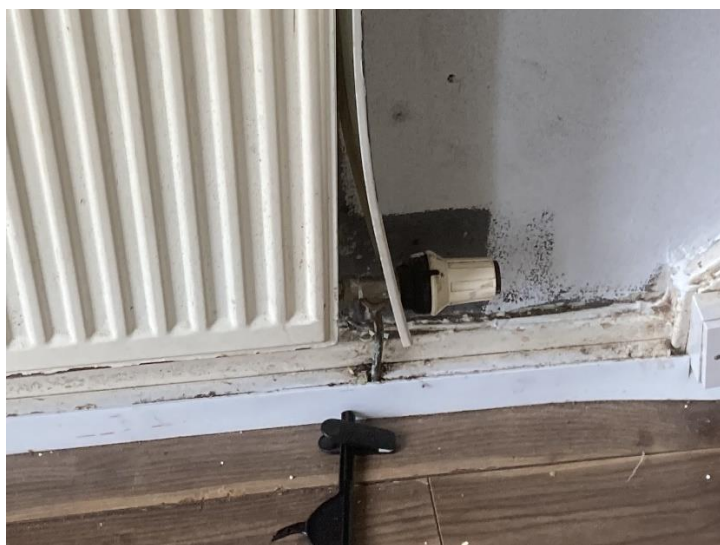
21. Broken radiator panel and condensation staining in hall
