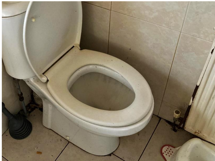
20. damp around base of wc and corroded radiator
