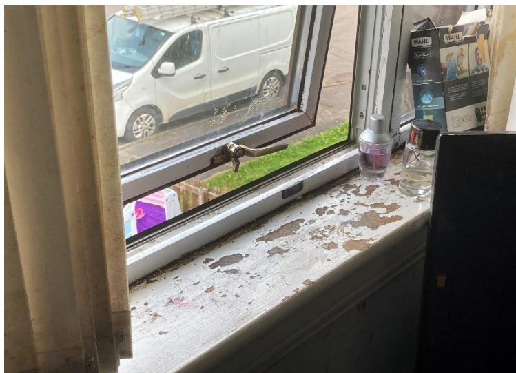
12. Condensation at front bedroom window
