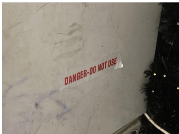
5. Gas boiler front casing
