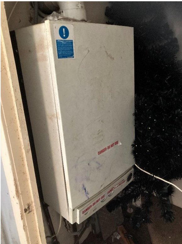
4. Wall mounted gas boiler
