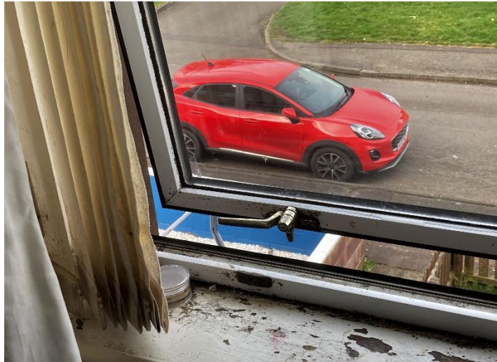
13. Condensation at front bedroom window
