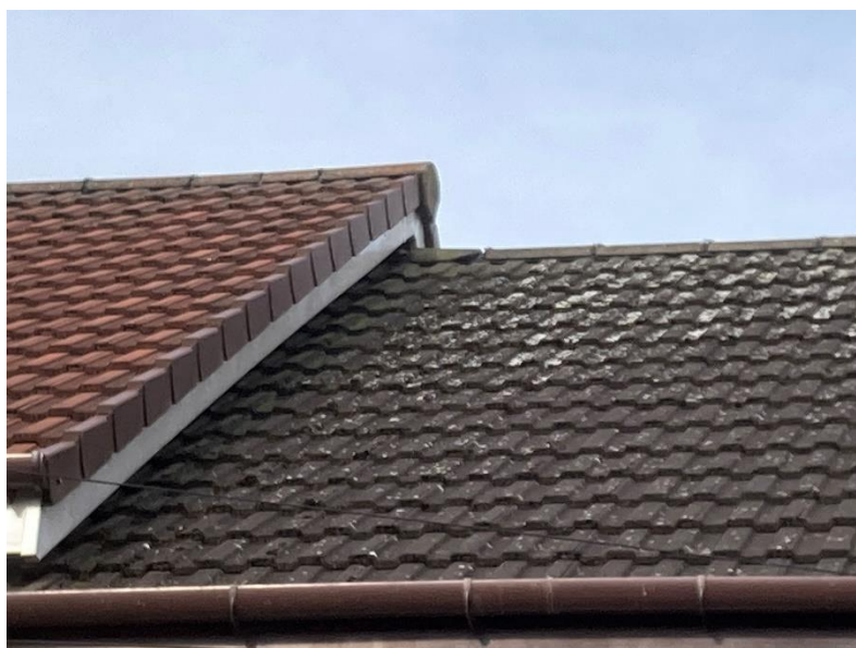
2. Rear roof pitch and ridge defective/slipped ridge tile
