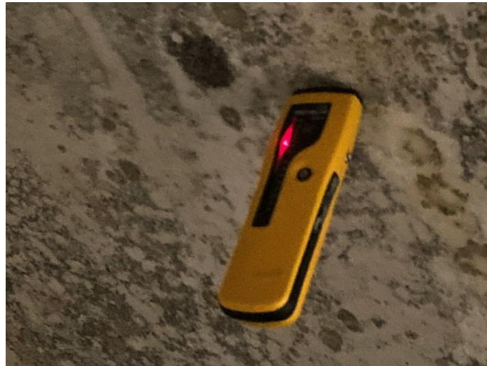
8. Damp "ceiling plaster" in attic
