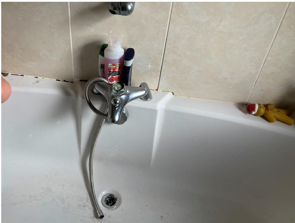
18. Broken mixer tap and "hand held" shower attachment
