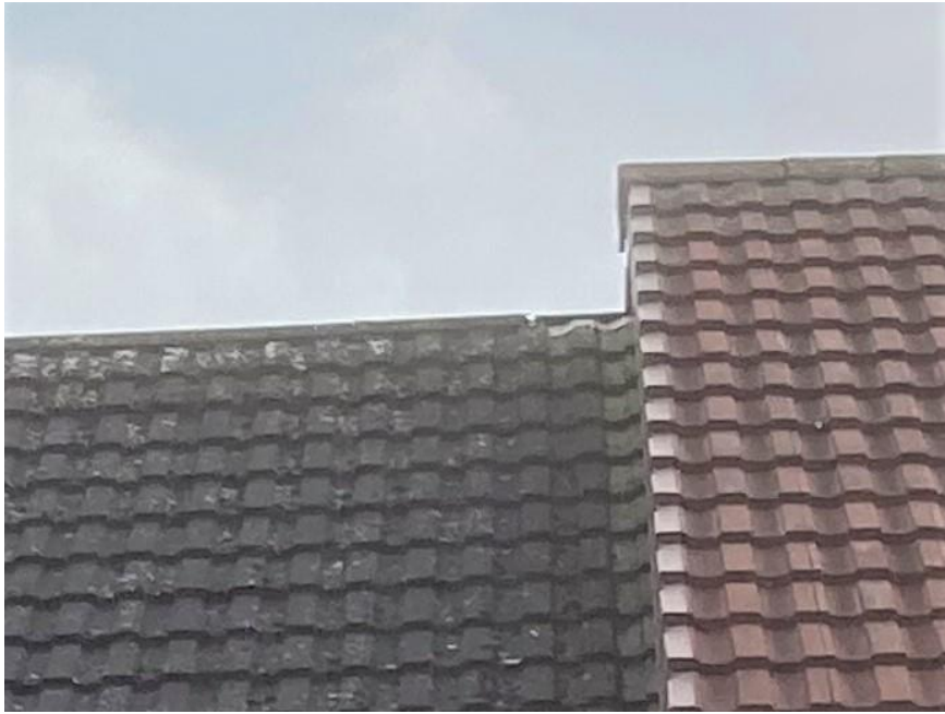
3. Front roof pitch and defective/slipped ridge tile.
