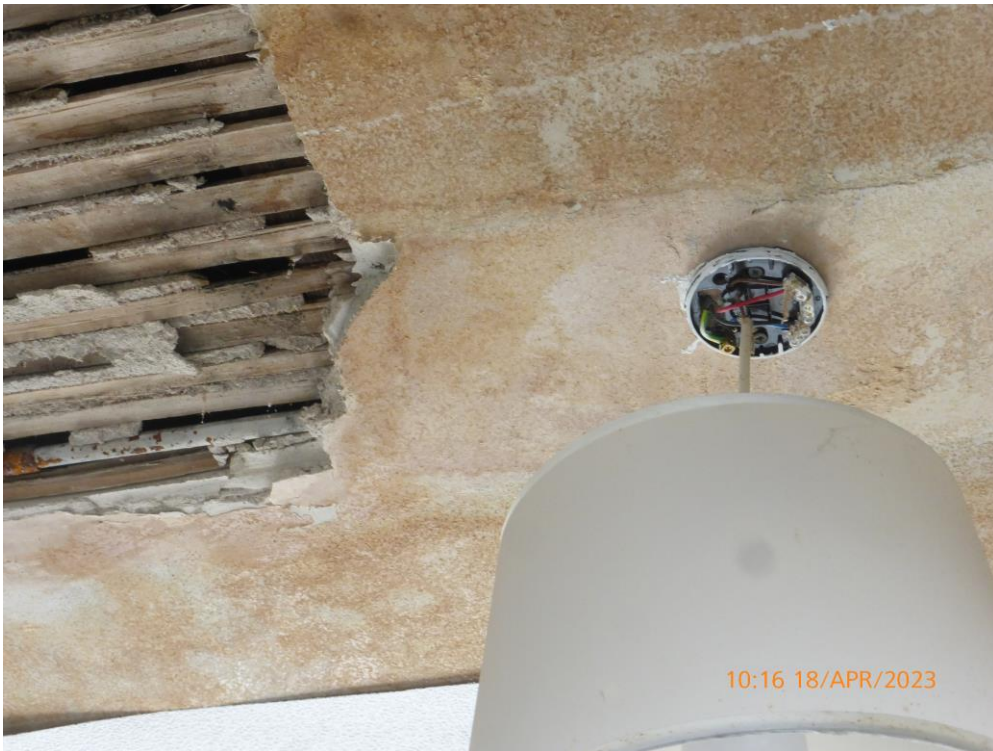
Exposed wiring and assumed metal conduit
