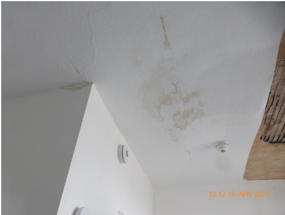
Additional affected areas in the kitchen
