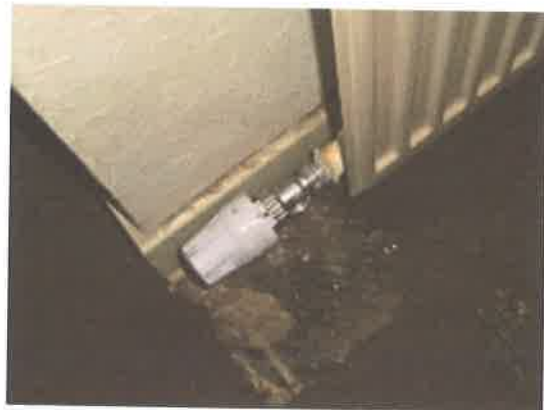
NEW VALVE – REAR BED RADIATOR
