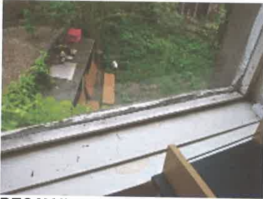
DECAY IN REAR BED WINDOW FRAME
