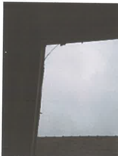
CRACKED PANE IN LR WINDOW
