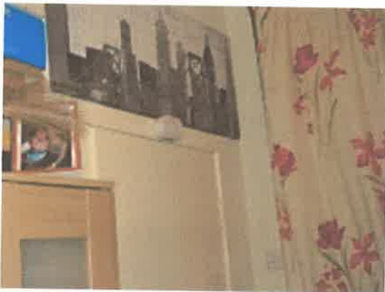
CO ALARM IN REAR BED
