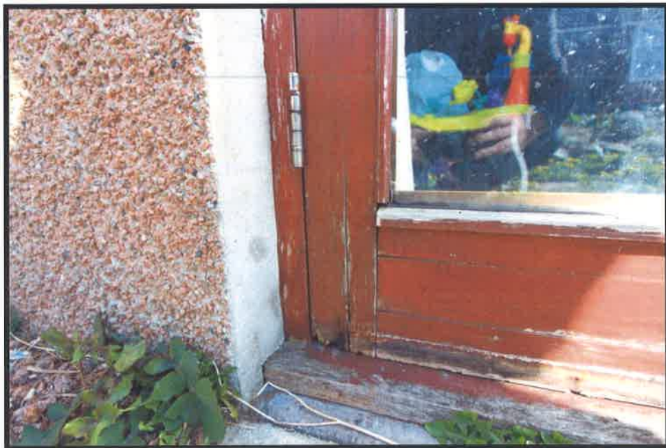
Figure 3 French Doors - decay and open joints.
