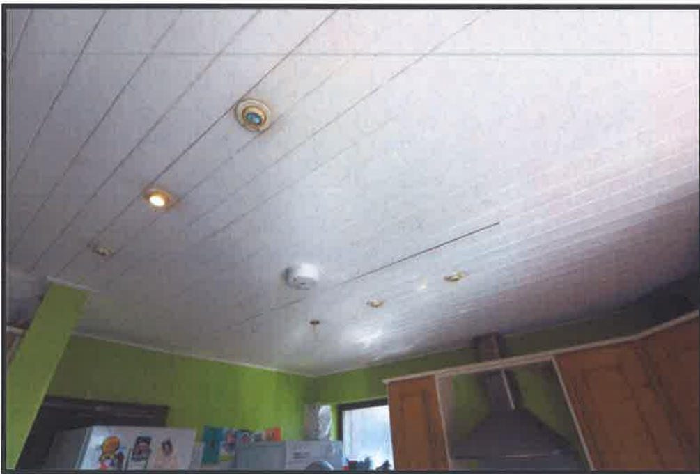
Figure 18 Kitchen Ceiling - Heat detector and lighting.
