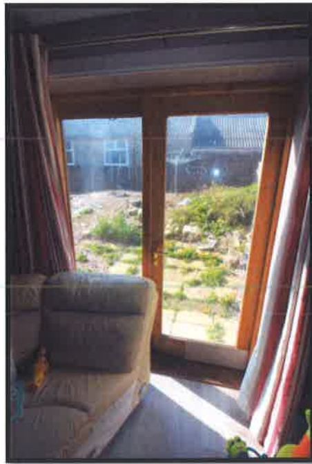
Figure 4 Lining Room French Doors internal - frame patched, misting to left pane.
