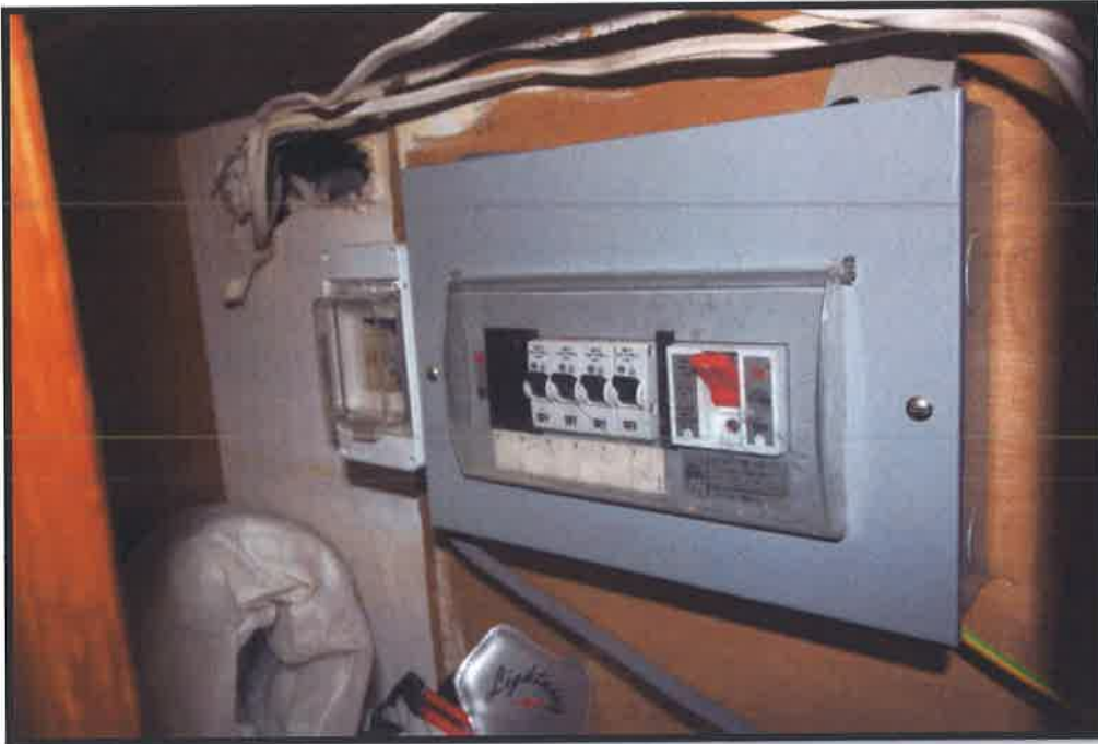
Figure 15 Electrical Switchgear (Left Hand).
