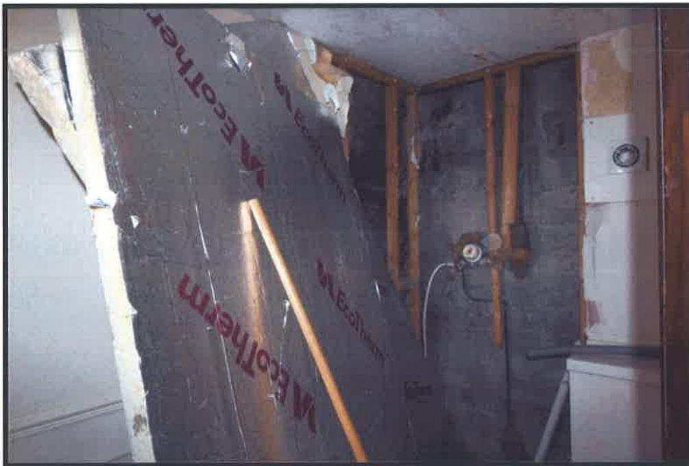
Figure 13 Main Shower Room - Shower enclosure missing, bare walls exposed.
