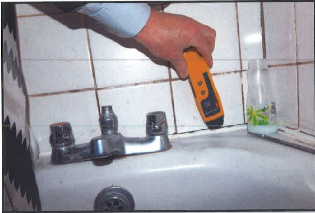
Figure 10 Main Bedroom bath - Moisture meter reading 81.9%/Red.
