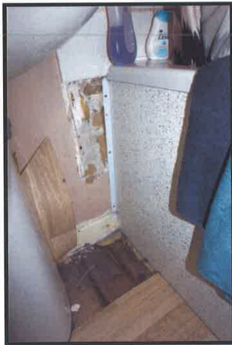
Figure 11 Main Bedroom bath - gaps sealed with silicon.
