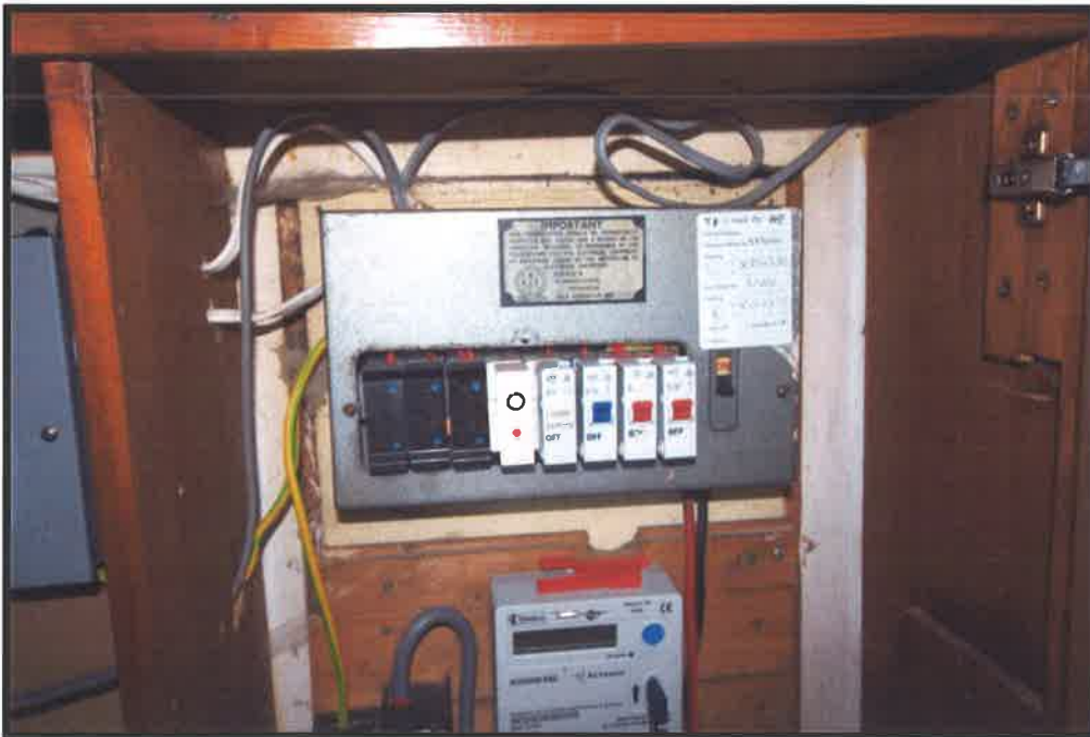
Figure 14 Electrical switchgear (Right Hand).
