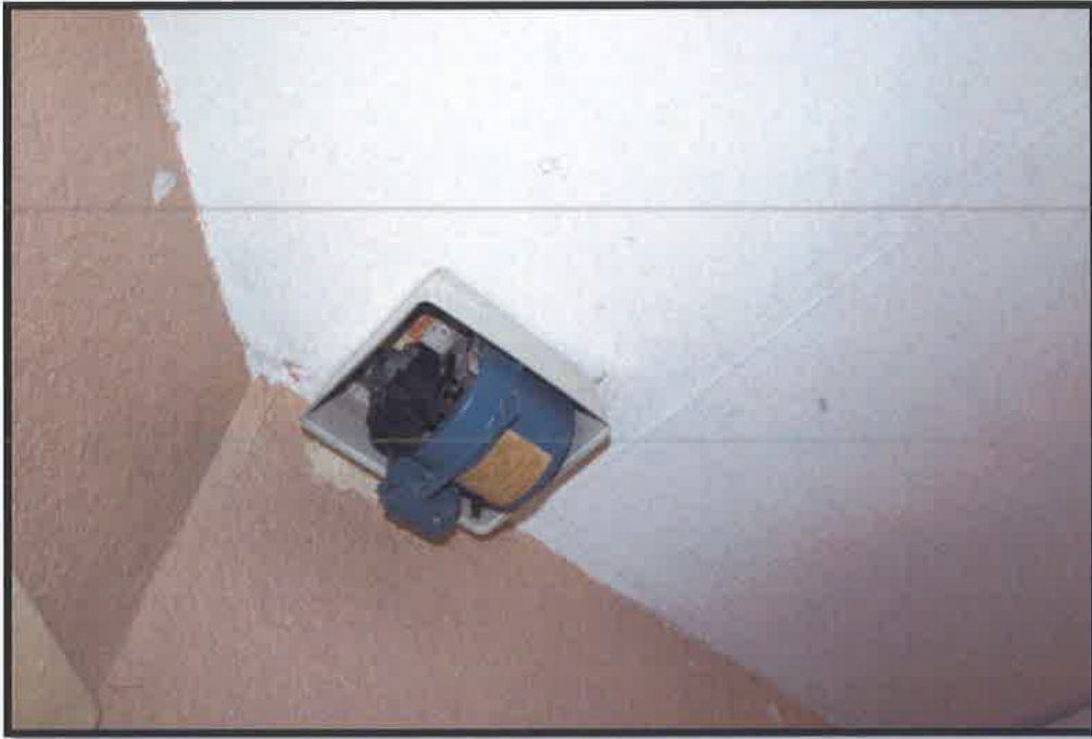
Figure 12 Main Bedroom Bathroom - extractor fan inoperative and cover removed.
