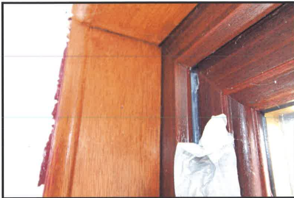
Figure 6 Main Bedroom window - gap at frame filled with silicon and duct tape
