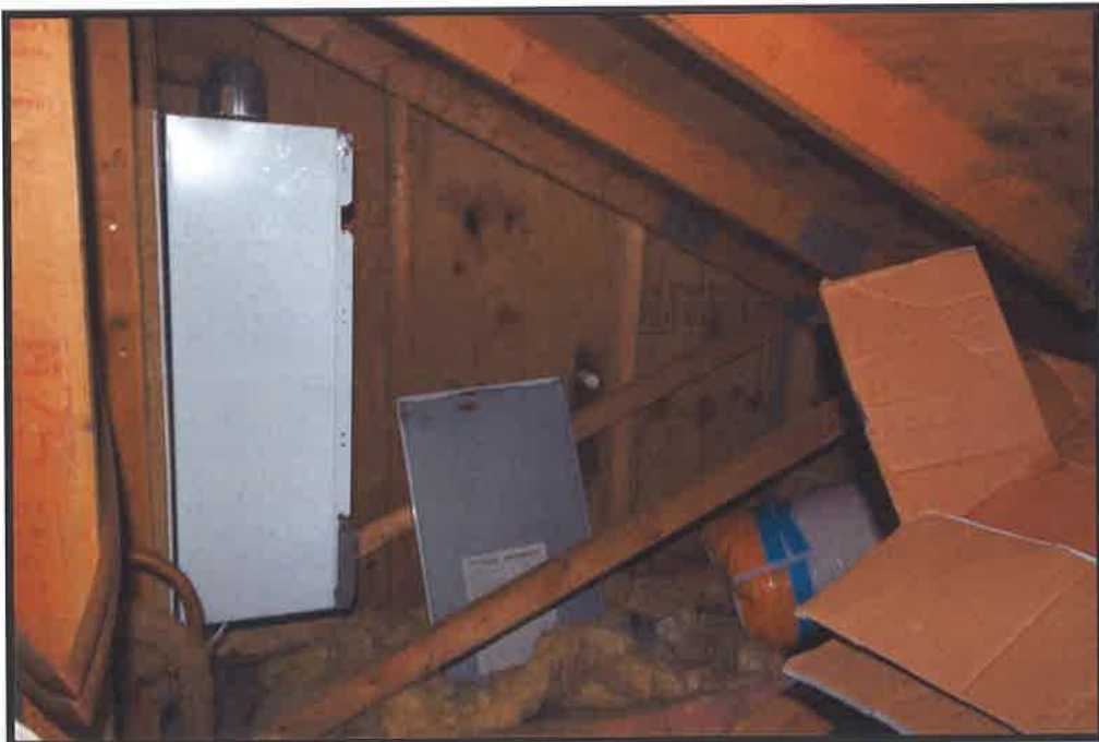
Figure 16 Central Heating boiler.
