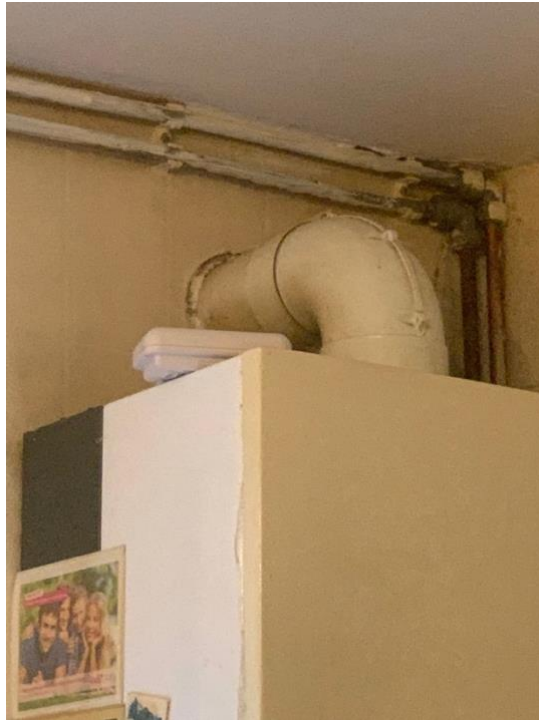
Photograph 4: Carbon monoxide detector laid on top of boiler
