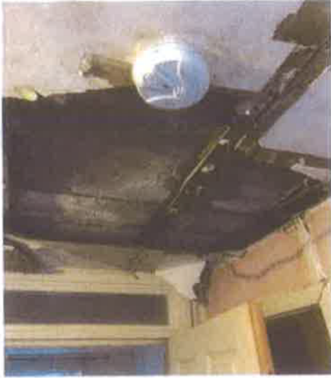
Photo 2 – Water damaged kitchen ceiling
