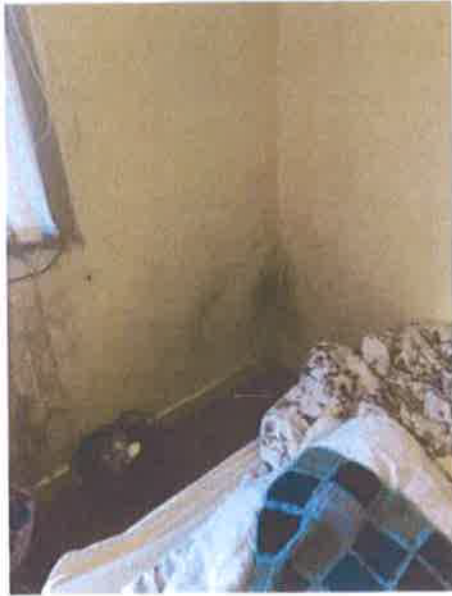
Photo 14 – Mould on wall in front bedroom
