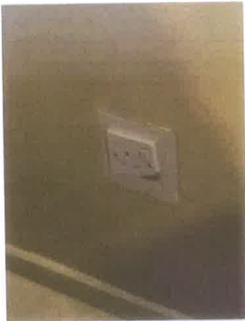
Photo 12 – Broken socket in Living Room
