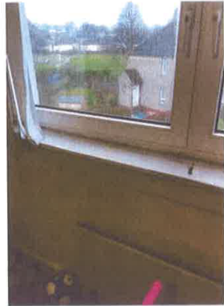
Photo 15 – More mould in same room
