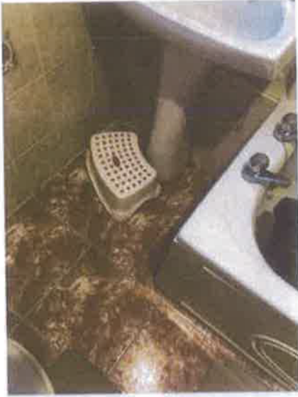
Photo 10 – Below surface dampness on floor
