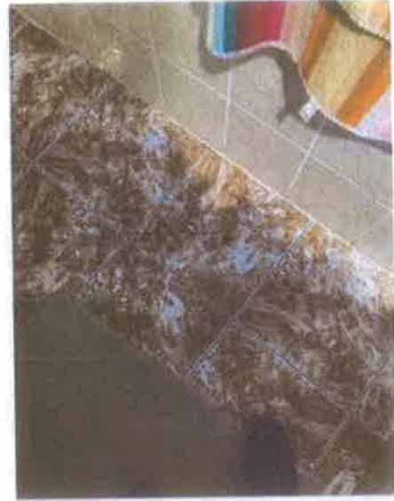
Photo 11 – Dampness beneath floor tiles
