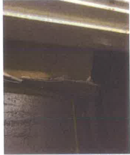
Photo 3 – Damaged cupboard ceiling
