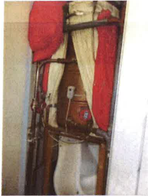
Upper landing cupboard - hot water tank
