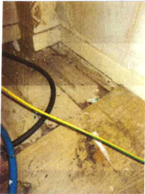
Kitchen - Exposed floorboards showing water staining
