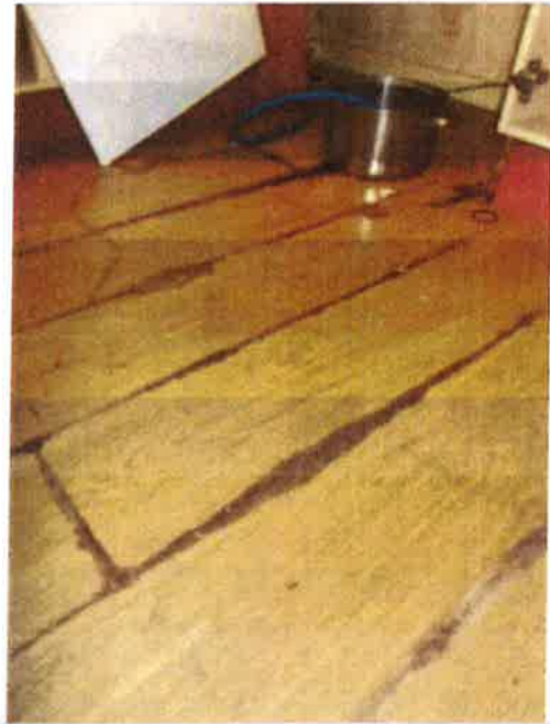
Kitchen - damaged laminate floor covering
