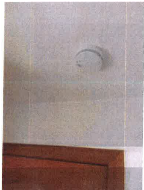
Lower Hall - ceiling mounted smoke alarm
