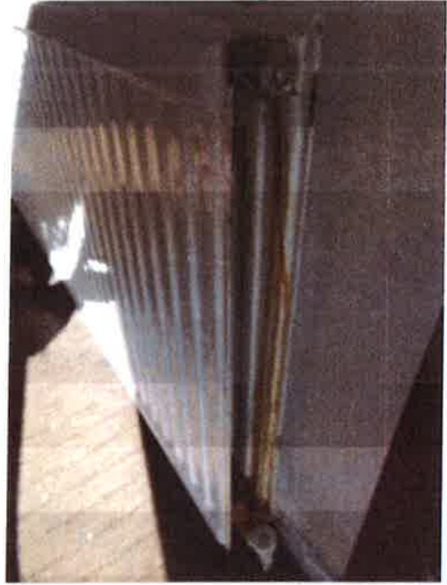
Living Room - radiator
