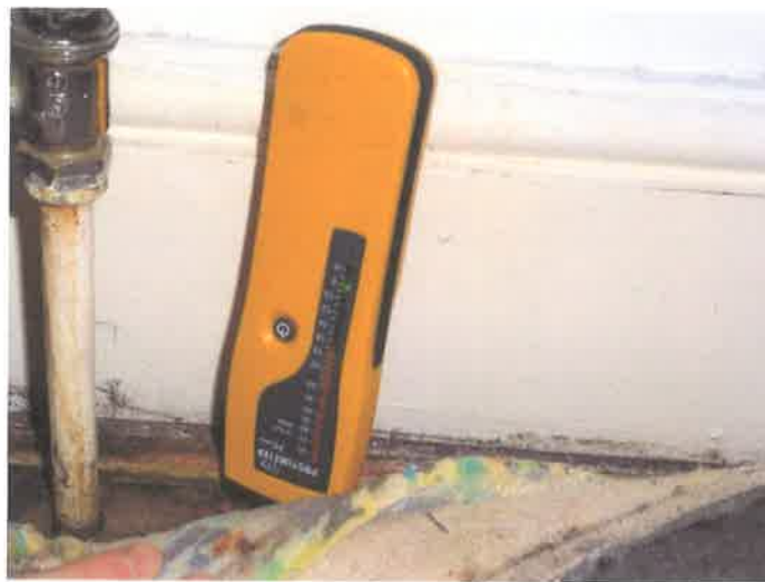
(9) No significant damp reading at rear bedroom radiator (8%)
