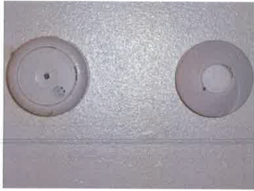
(6) Heat / smoke detectors hall
