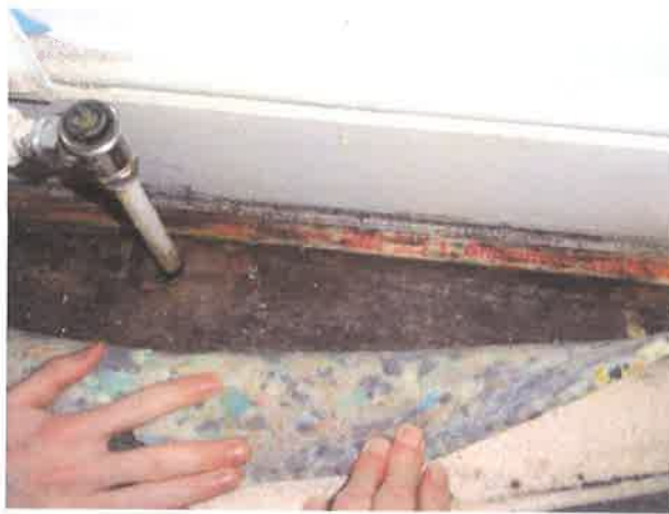
(8) Old Damp staining at rear bedroom radiator
