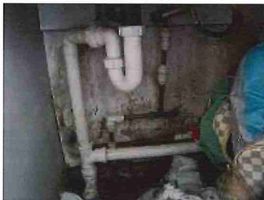
DAMP BENEATH SINK
