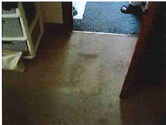
UNEVEN FLOORING IN BEDROOM
