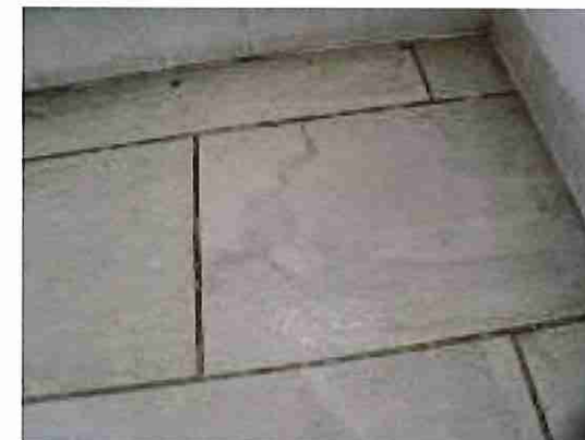
DAMP ON KITCHEN FLOOR
