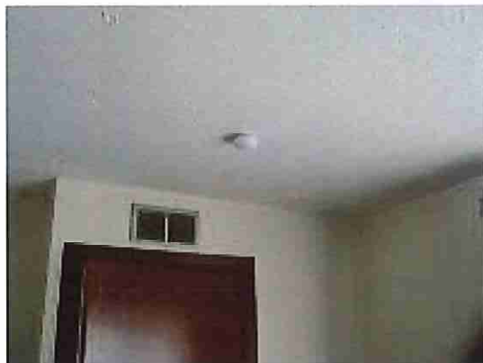
LIVING ROOM – SMOKE DETECTOR
