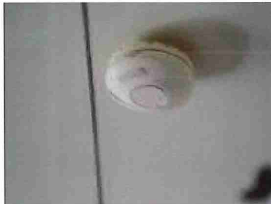
KITCHEN – SMOKE/HEAT DETECTOR
