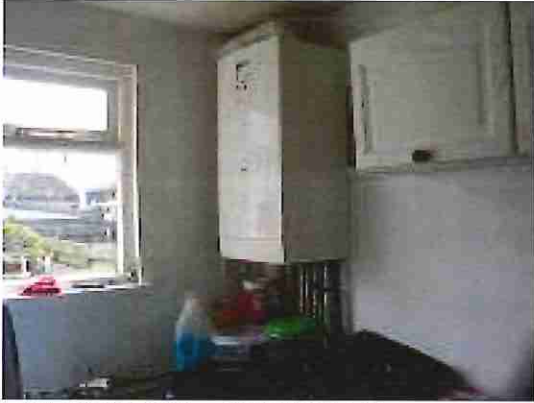
UTILITY ROOM – GAS BOILER
