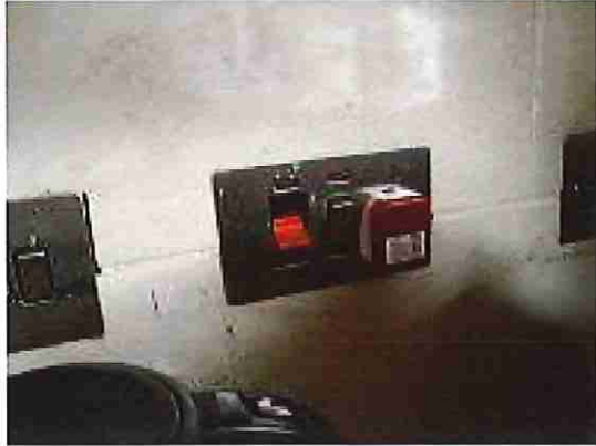
KITCHEN SOCKET-NOT WORKING
