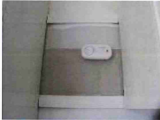
CO MONITOR ADJACENT TO BOILER
