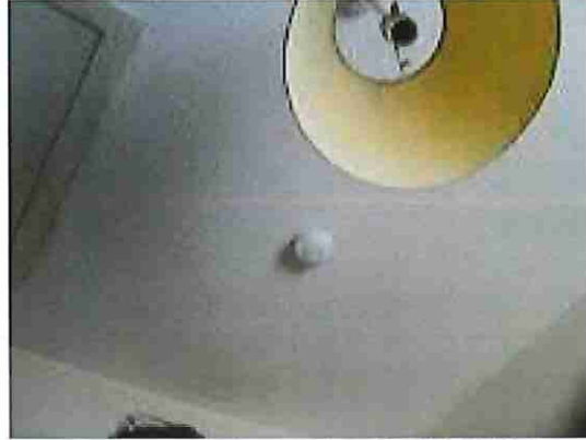
LANDING CEILING SMOKE DETECTOR
