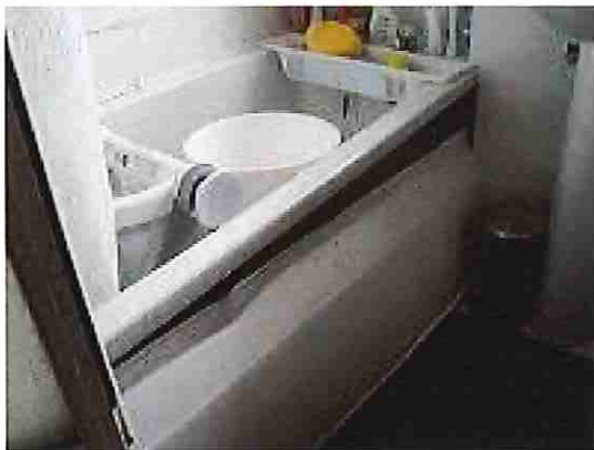
BROKEN BATH PANEL
