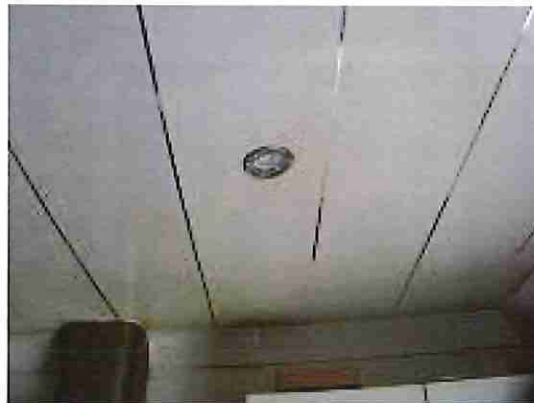
LEAK IN KITCHEN CEILING AT LIGHT
