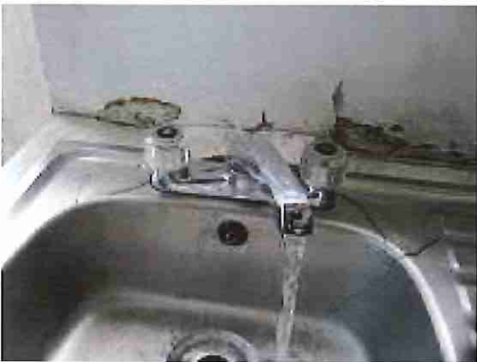
UTILITY ROOM SINK – TAPS LEAKING
