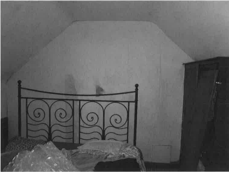
Observation – 2 nd floor bedroom gable wall very damp.
