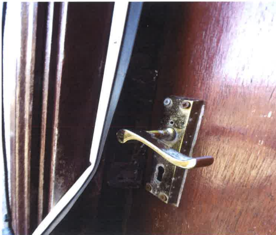
Door catch and latch do not meet because door frame split, lock loose and unsafe.
