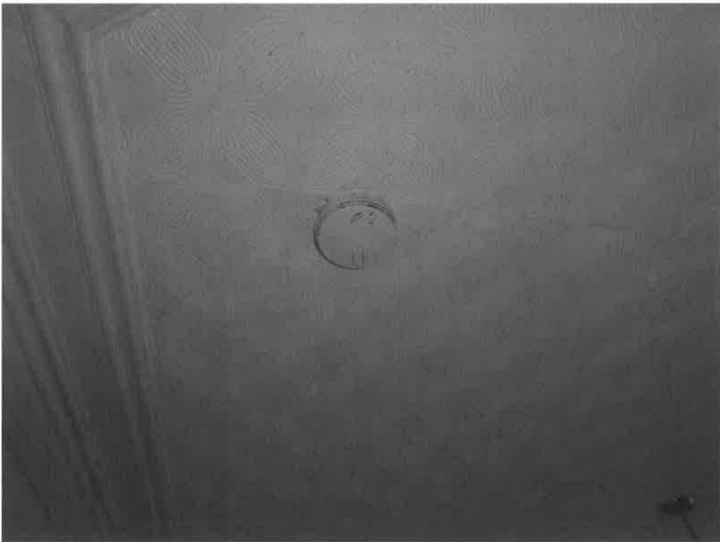
Smoke alarm on living room ceiling
