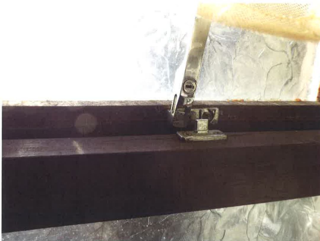
Bathroom window does not close.
