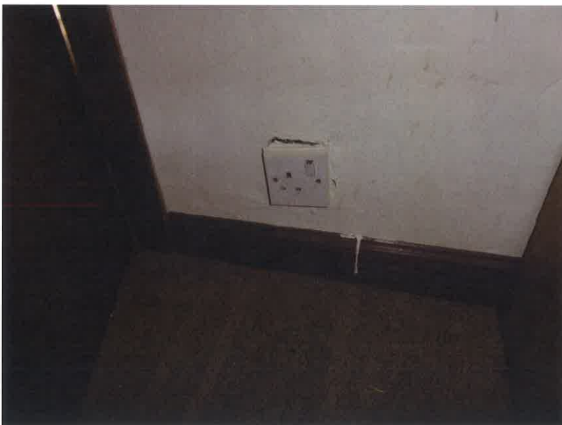
Bedroom socket in disrepair.
