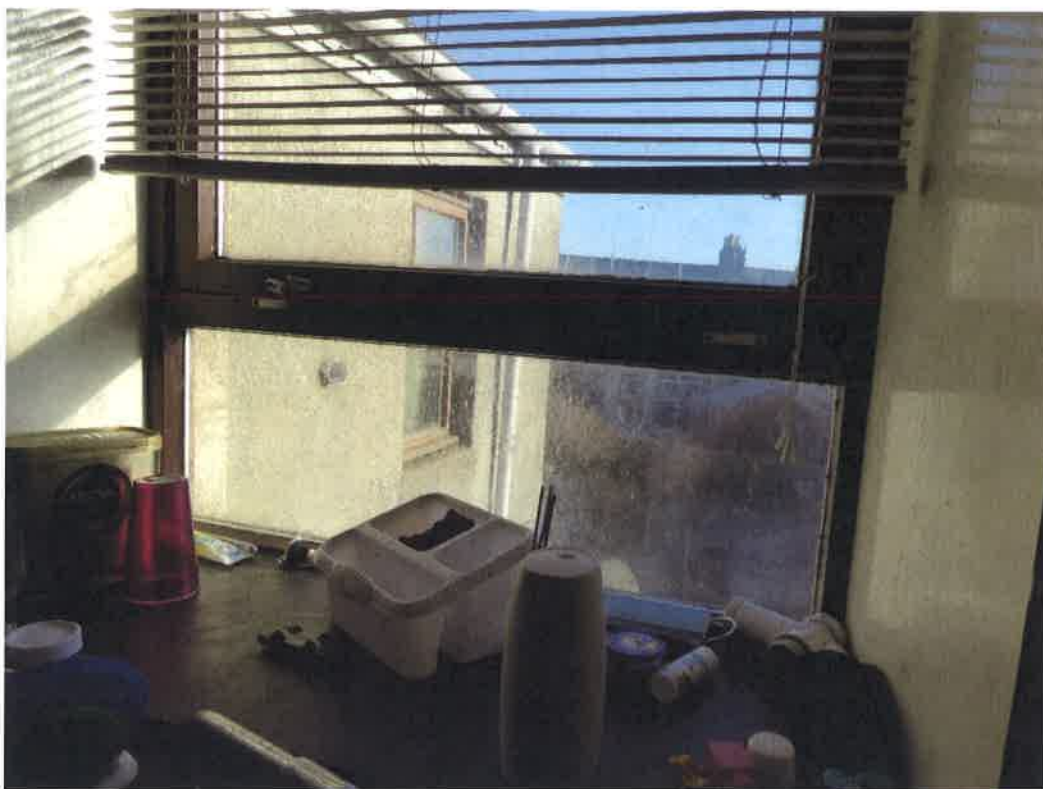
Kitchen windows. No handles to operate catches to window.
