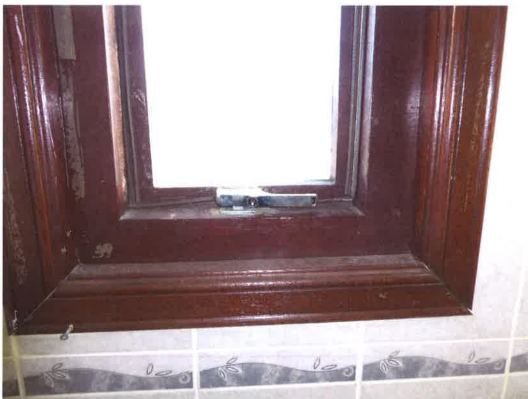
Bathroom window – locked shut
