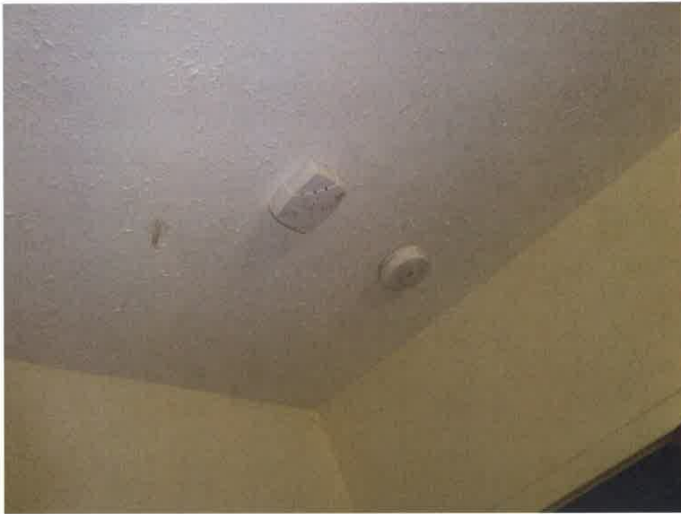
Heat and CO detectors on kitchen ceiling
