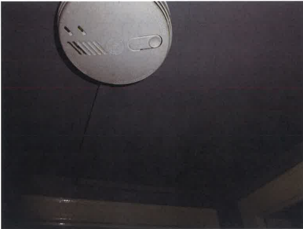
Smoke alarm on landing ceiling to 2nd floor.
