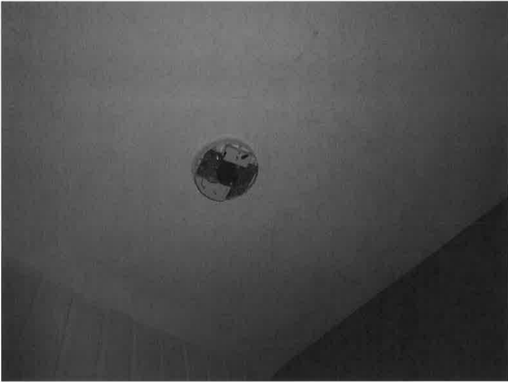
Damaged smoke alarm on corridor ceiling
