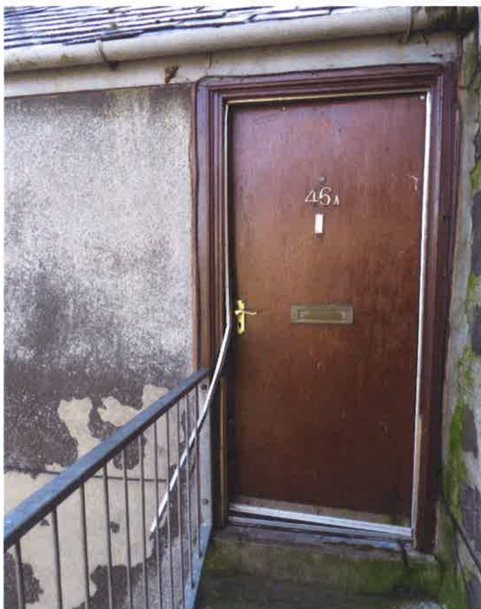
Door to flat does not open or close properly. Draught proof strip partly unfixed and bent out of shape.
