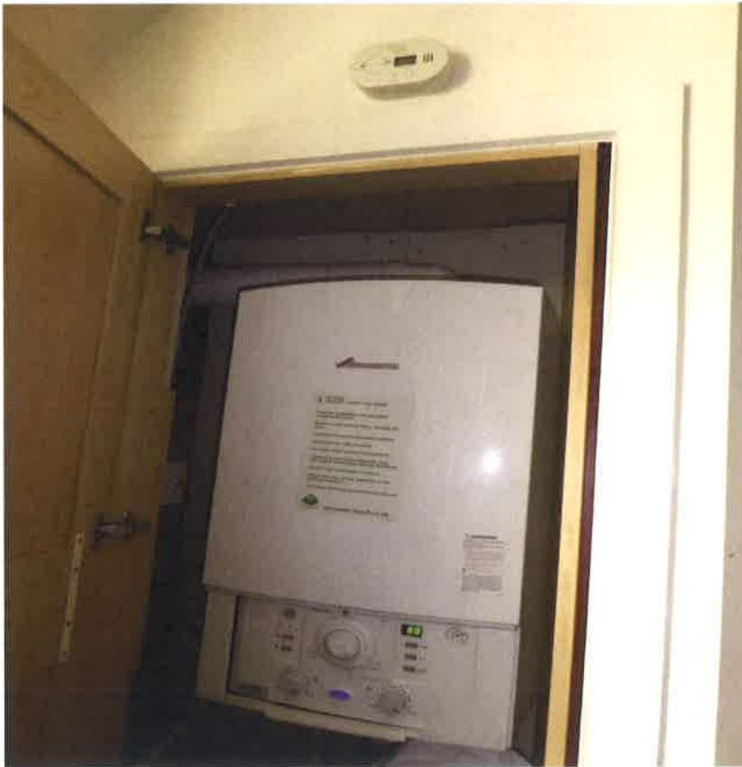
CO alarm above boiler (too close – should be 1m + away)
