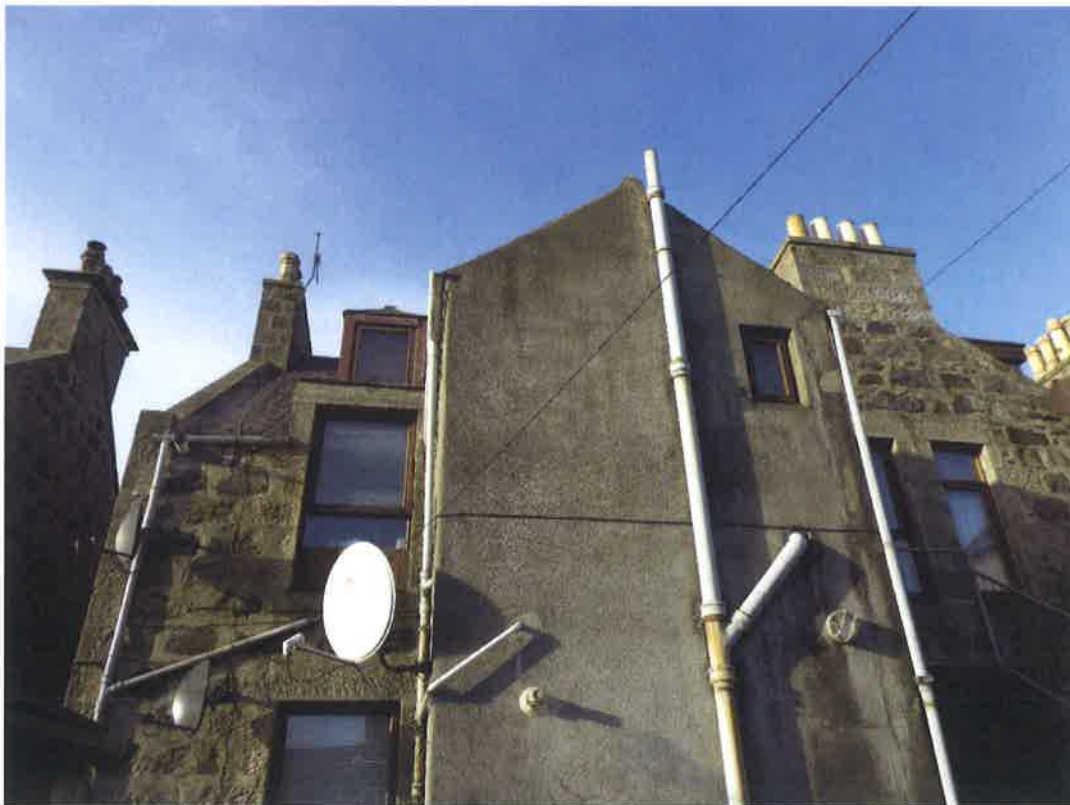
Rear elevation – 1 st & 2 nd floors. Left hand window to kitchen. Extension window to bathroom.
