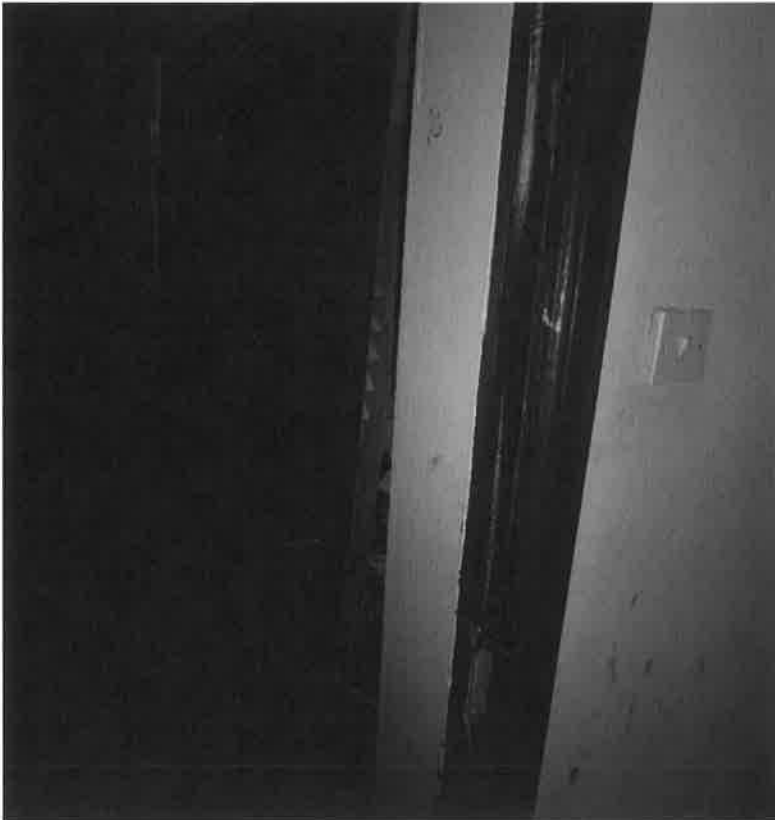
Observation – cupboard door on 2 nd floor and cupboard door on 1 st floor off their hinges
