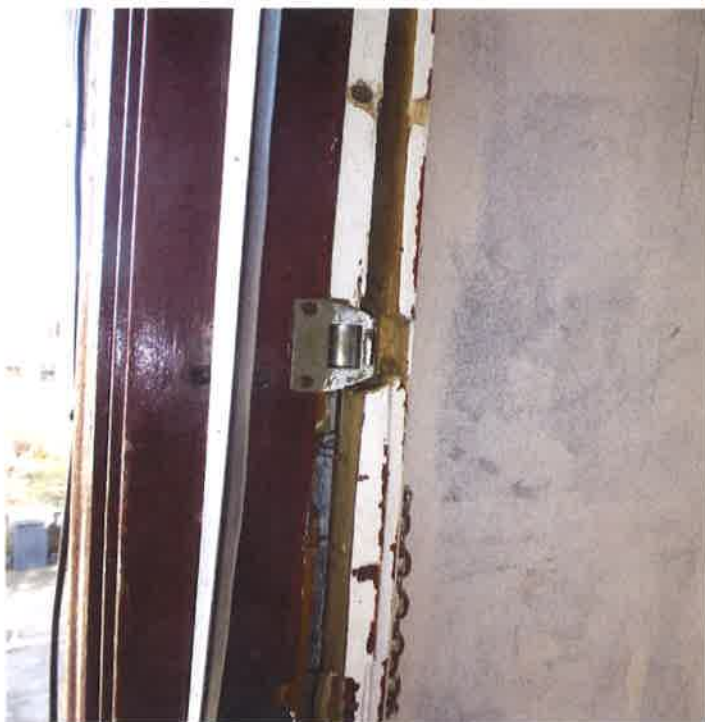
Internal view of split door frame above door catch.
