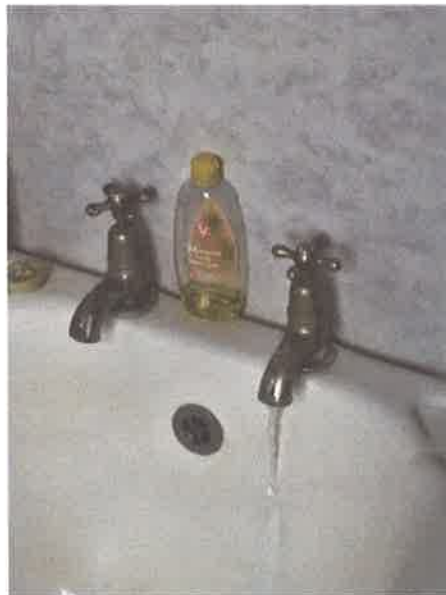
16. Water flow from cold tap when in off position
