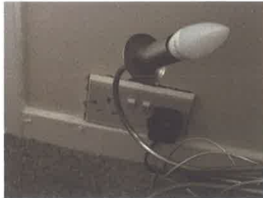
11. Living room double electrical socket
