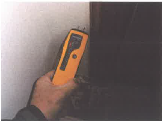
4. Damp internal wall at front door
