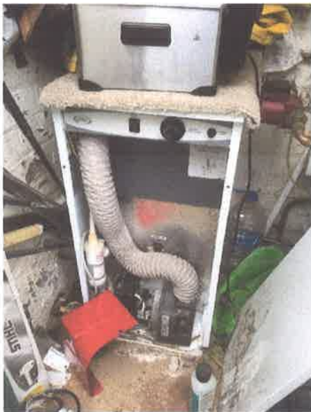
15. Oil fired "Grant Vortex Eco Utility" boiler (functional) in outhouse
