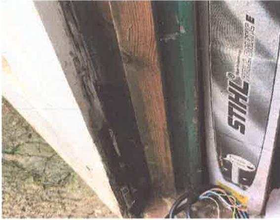
6. Defective hinge & rot at boiler house door
