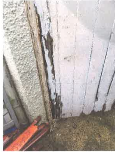
7. Rotted boiler-house door
