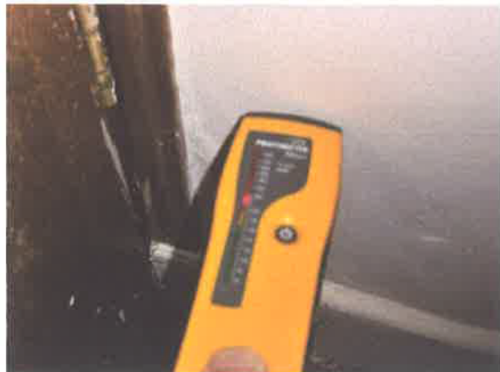
5. Damp internal wall at front door
