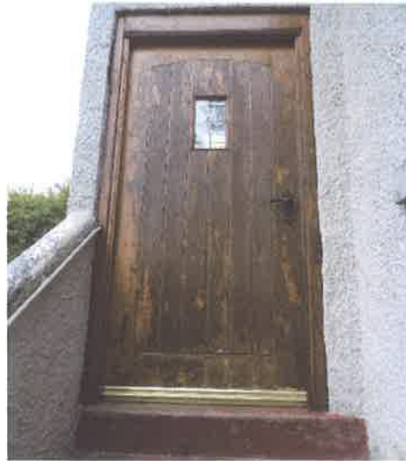
3. External face front door
