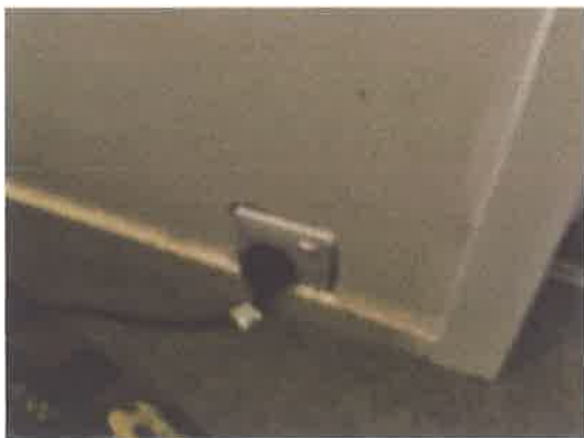
10. Hall single electrical socket
