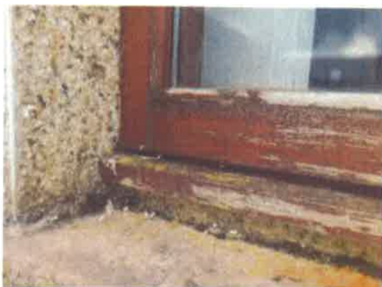
31 Ground Floor bedroom – missing perimeter sealant.
