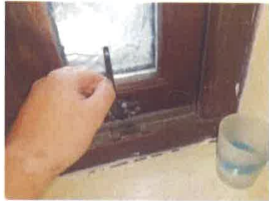
8 Loose handle ironmongery to WC window.
