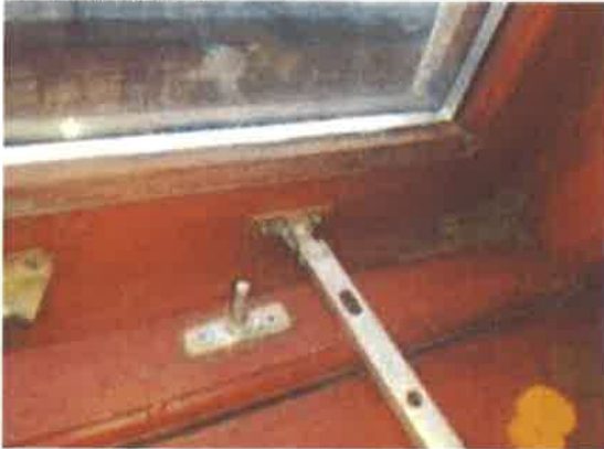
3 Ground Floor bedroom – binding in frame and operation impaired.
