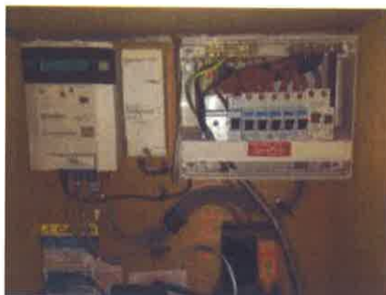
38 Consumer unit – front cover not secured and “risk of death” due to uncontrolled access to “live” cables.
