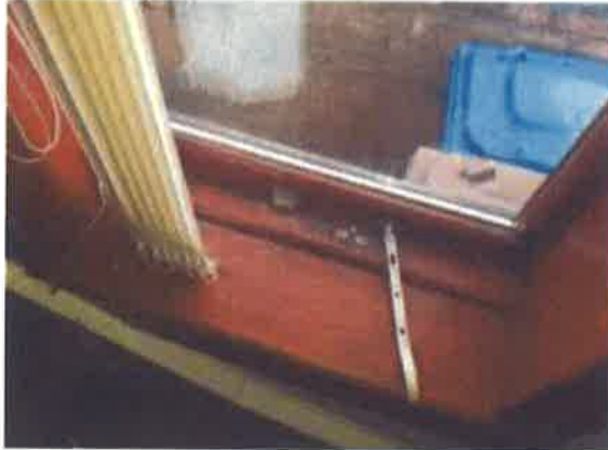
9 Stair window – binding in frame and operation impaired.
