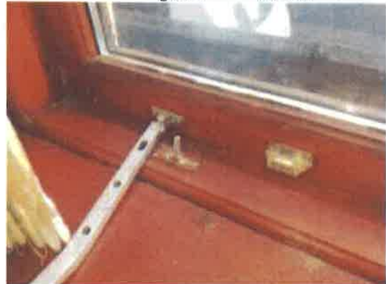
4 Ground Floor bedroom – binding in frame and operation impaired.
