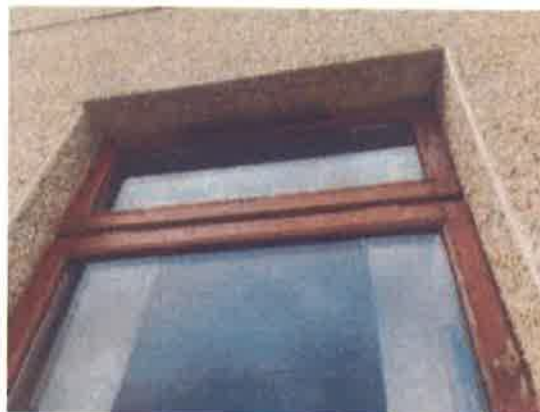
32 Ground Floor bedroom – missing perimeter sealant.
