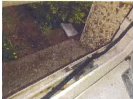
2 Defective and loose gasket seal to Kitchen window.
