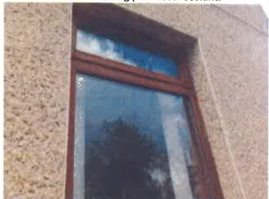
28 Ground Floor Bedroom – missing perimeter sealant.
