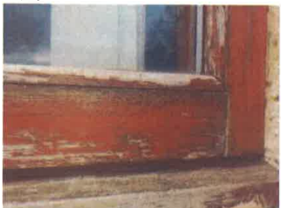
30 Ground Floor Bedroom - poor paint finish generally to windows and missing perimeter sealant.
