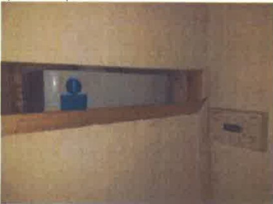
5 Ground Floor Bedroom – boiler.
