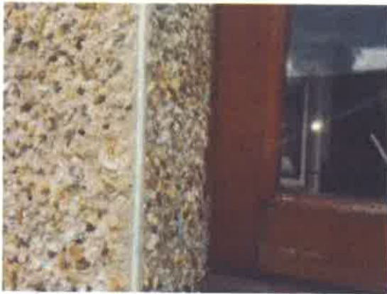
25 Stair window – missing perimeter sealant.
