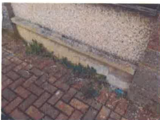
39 Defective smooth cement render base course below Living Room window.
