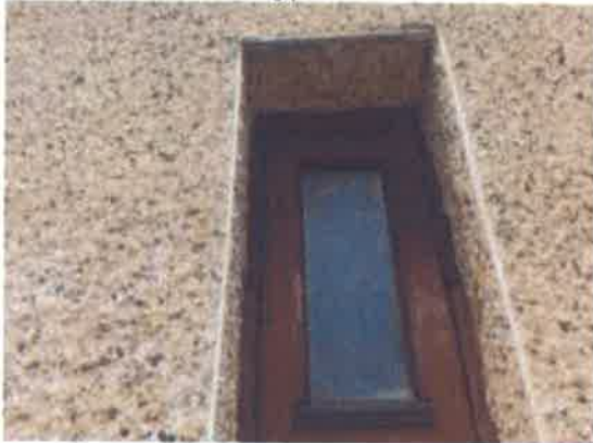
27 Cloakroom window – missing perimeter sealant.
