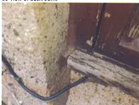
18 Timber decay at sill of living room and defective seals.
