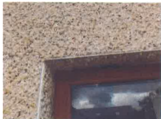
24 Stair window – perimeter seals not provided at junction between frame and ingoes.
