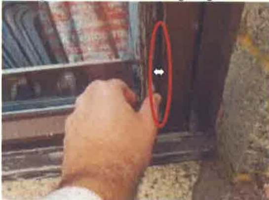
21 Living Room window – defective and loose glazing beads.
