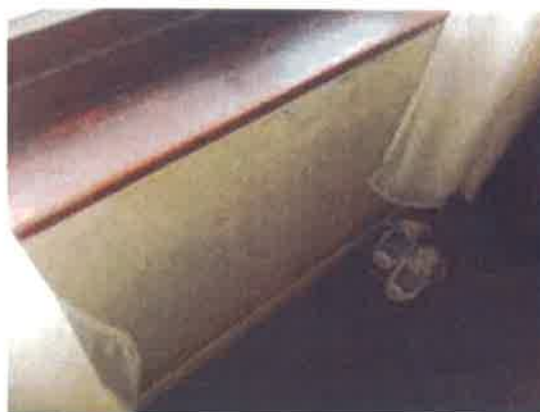
14 Plaster below Front Bedroom right hand window.
