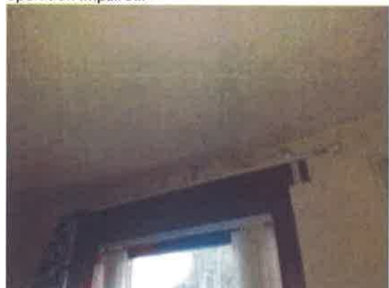
6 Staining above ground floor bedroom window.
