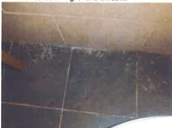
15 Bathroom – mould growth complaint.
