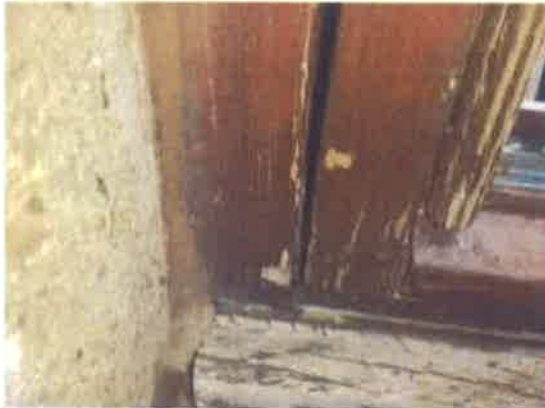
19 Living Room window – defective glazing beads.
