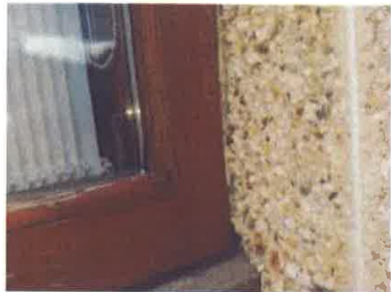
26 Stair window – missing perimeter sealant.
