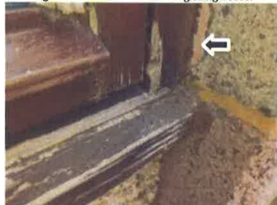
22 Living Room window – defective perimeter seals.
