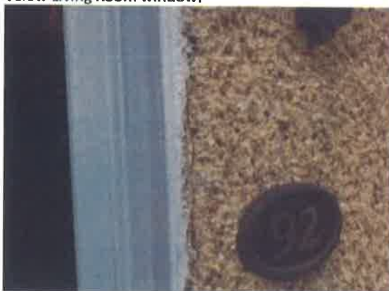
41 Cracking to render adjacent to entrance door.
