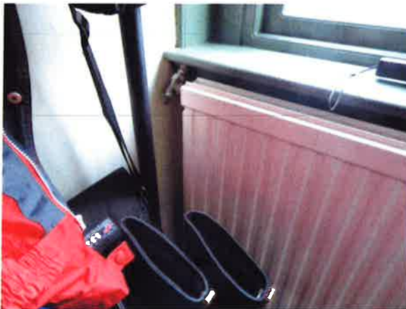
Photograph 2 :- Ground floor hall radiator with missing control valve.
