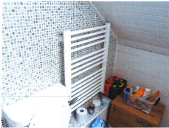
Photograph 5 :- First floor shower room radiator. Visible valve fitted. Radiator "tepid".
