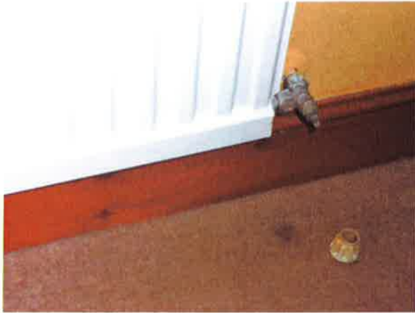
Photograph 4 :- Broken and defective / leaking valve at dining room radiator.
