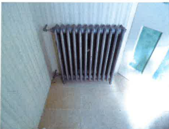
Photograph 3 :- Ground floor bathroom radiator with missing control valve.
