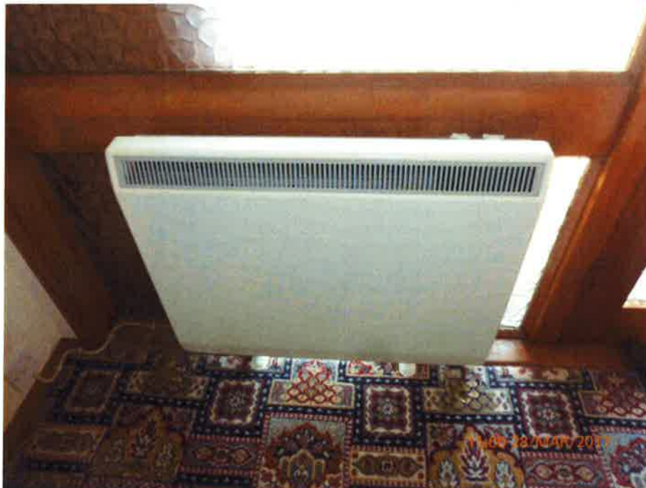
New storage heater
