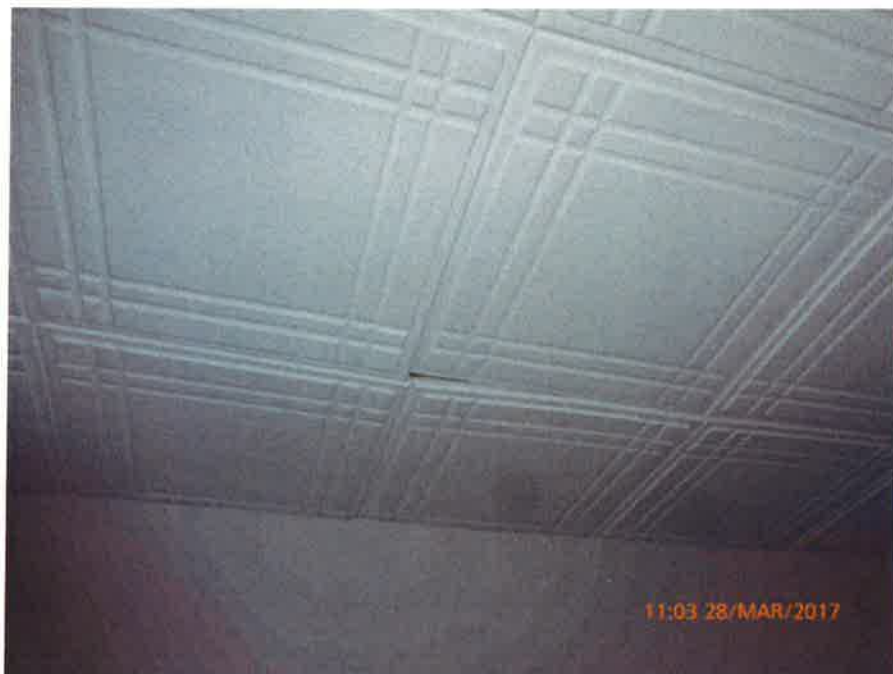
Loose ceiling tiles in the bathroom
