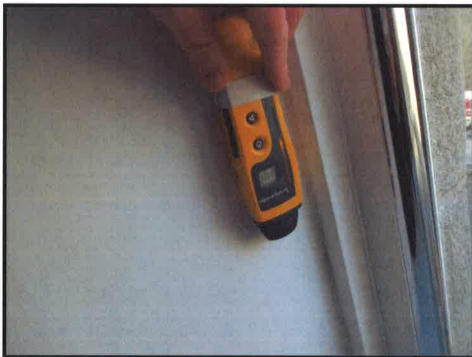
Figure 5 Further meter reading (20%) LHS lounge window, low level.
