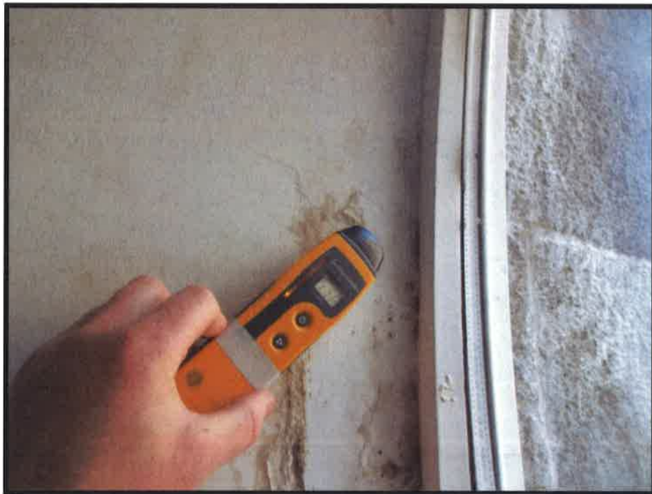
Figure 4 Meter reading (18%) and staining left hand side (LHS) lounge window
