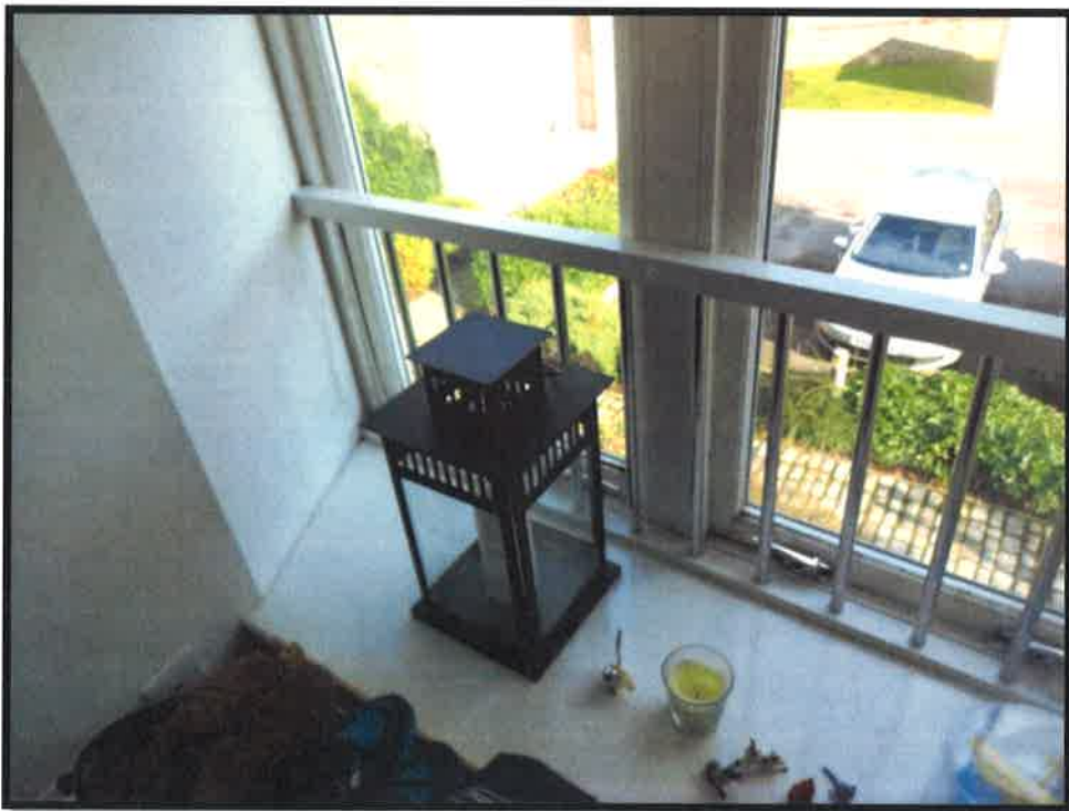
Figure 7 Master bedroom - mould growth to window frame
