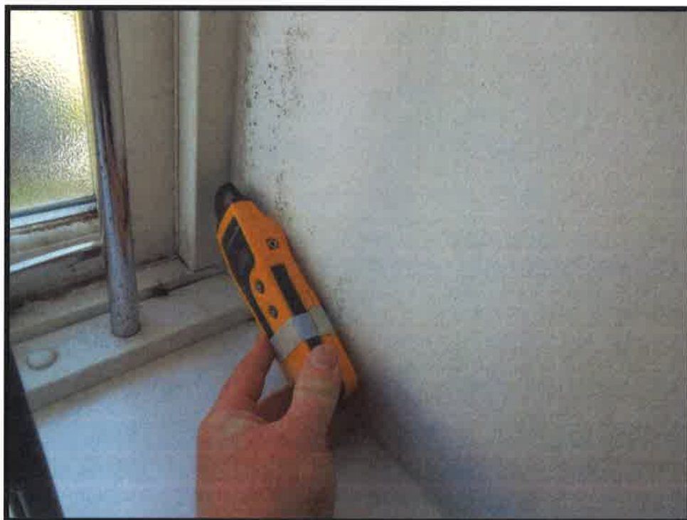
Figure 11- En-suite shower room - Mould to window ingo and frame
