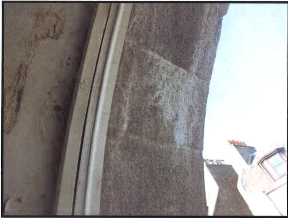
Figure 6 Efflorescence LHS lounge/kitchen window
