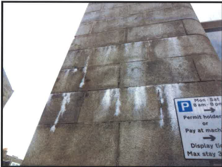
Figure 7 Front elevation - further efflorescence and missing pointing
