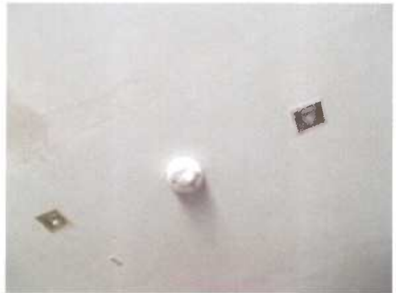
Heat alarm - Kitchen
