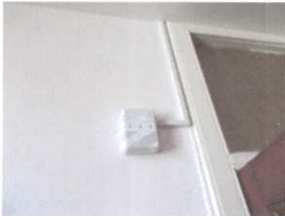
CO alarm - Kitchen
