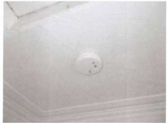
Smoke alarm - top landing
