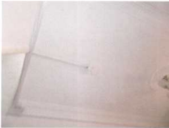
Smoke alarm - lower hall
