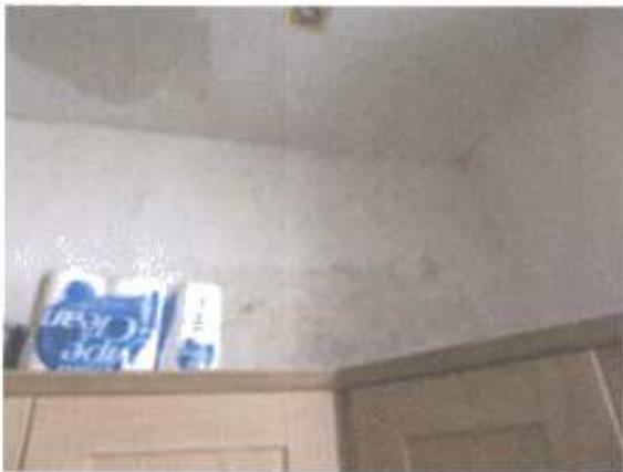
Kitchen ceiling and wall above fitted units
