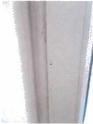
Living Room - Bay window - left - screw holes
