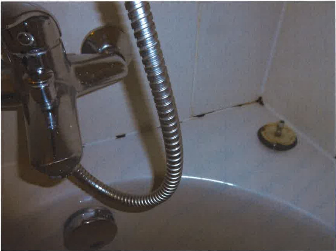
Mould around bath sealant
