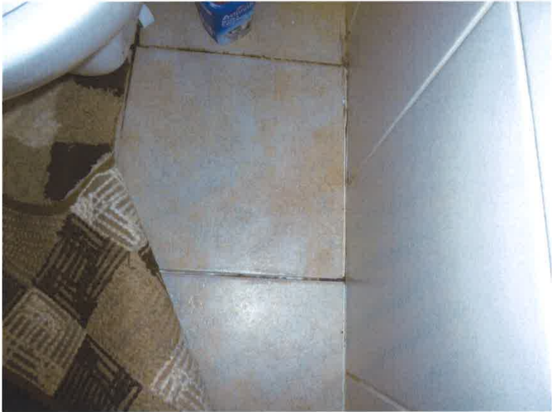
Mould on bathroom tiles
