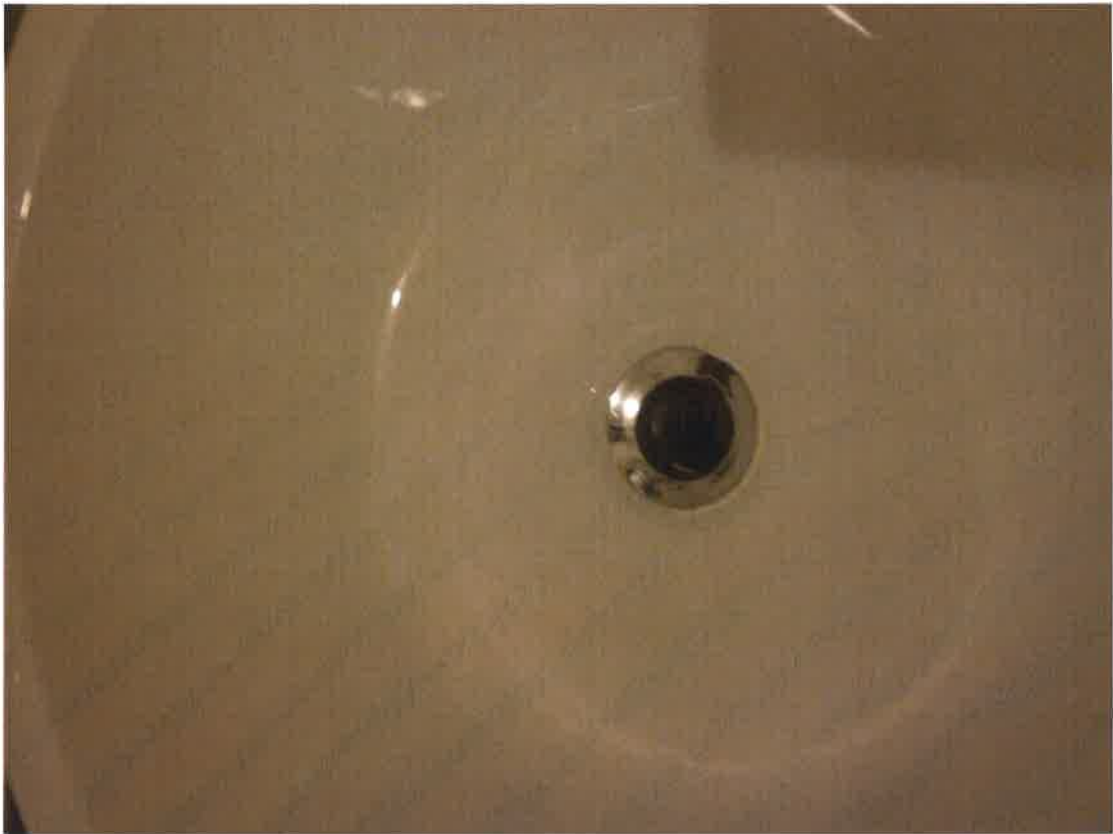
Cracked cloakroom sink
