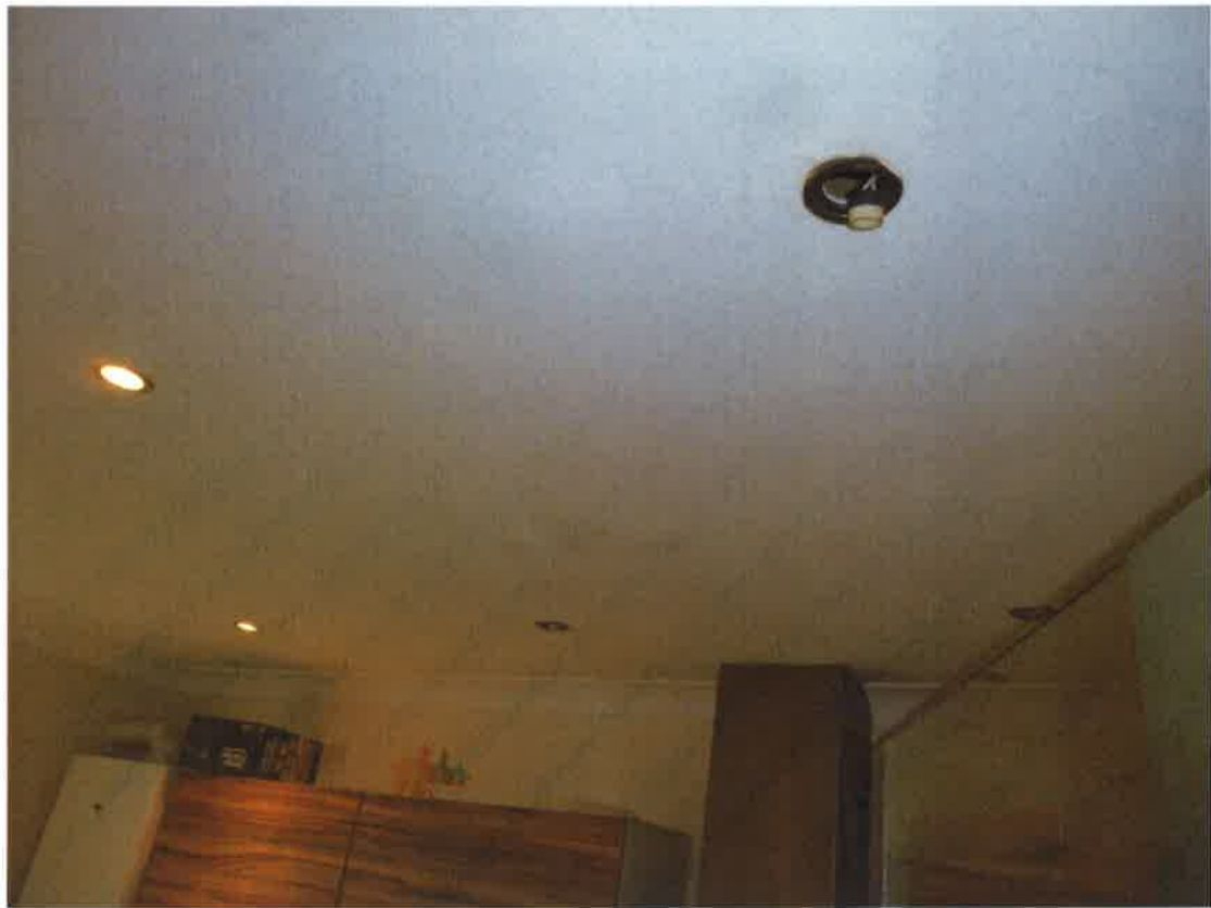
Kitchen ceiling/missing and damaged light socket
