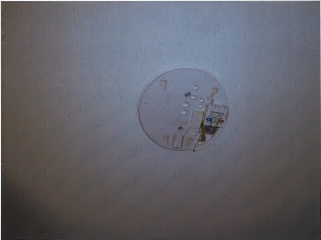
Downstairs hall – damaged smoke alarm
