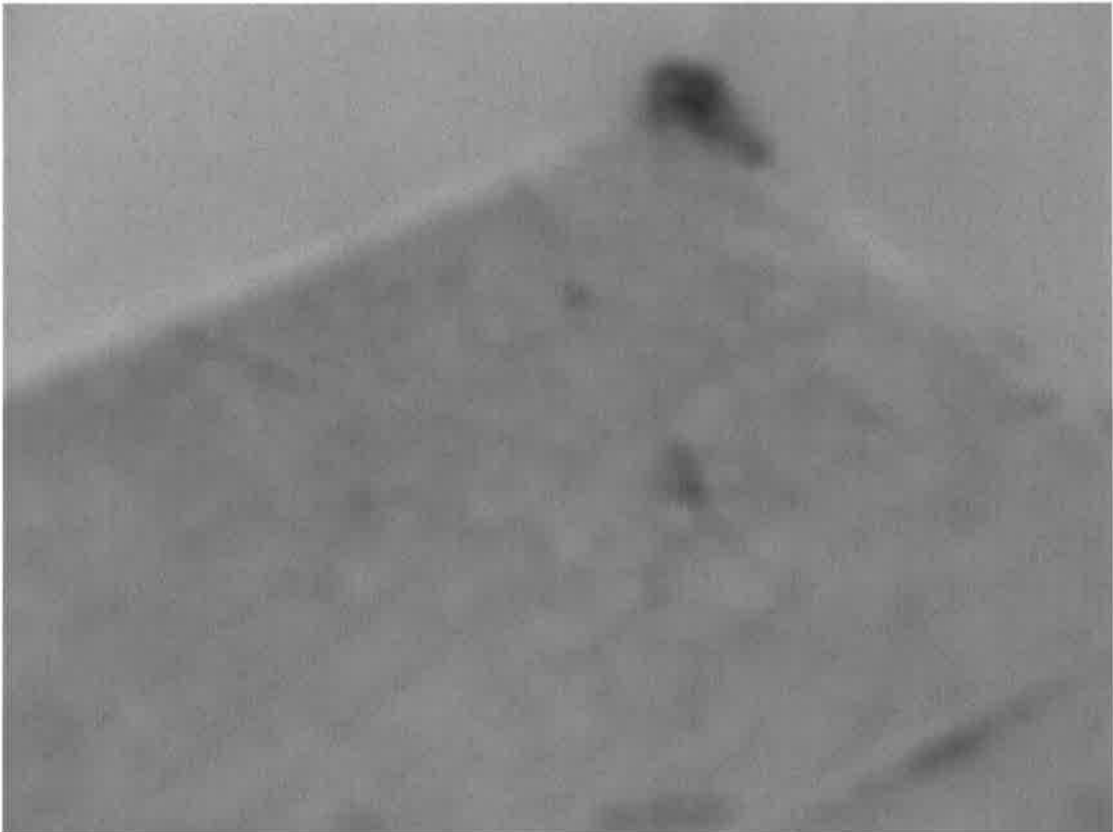
Cracked corner floor tile
