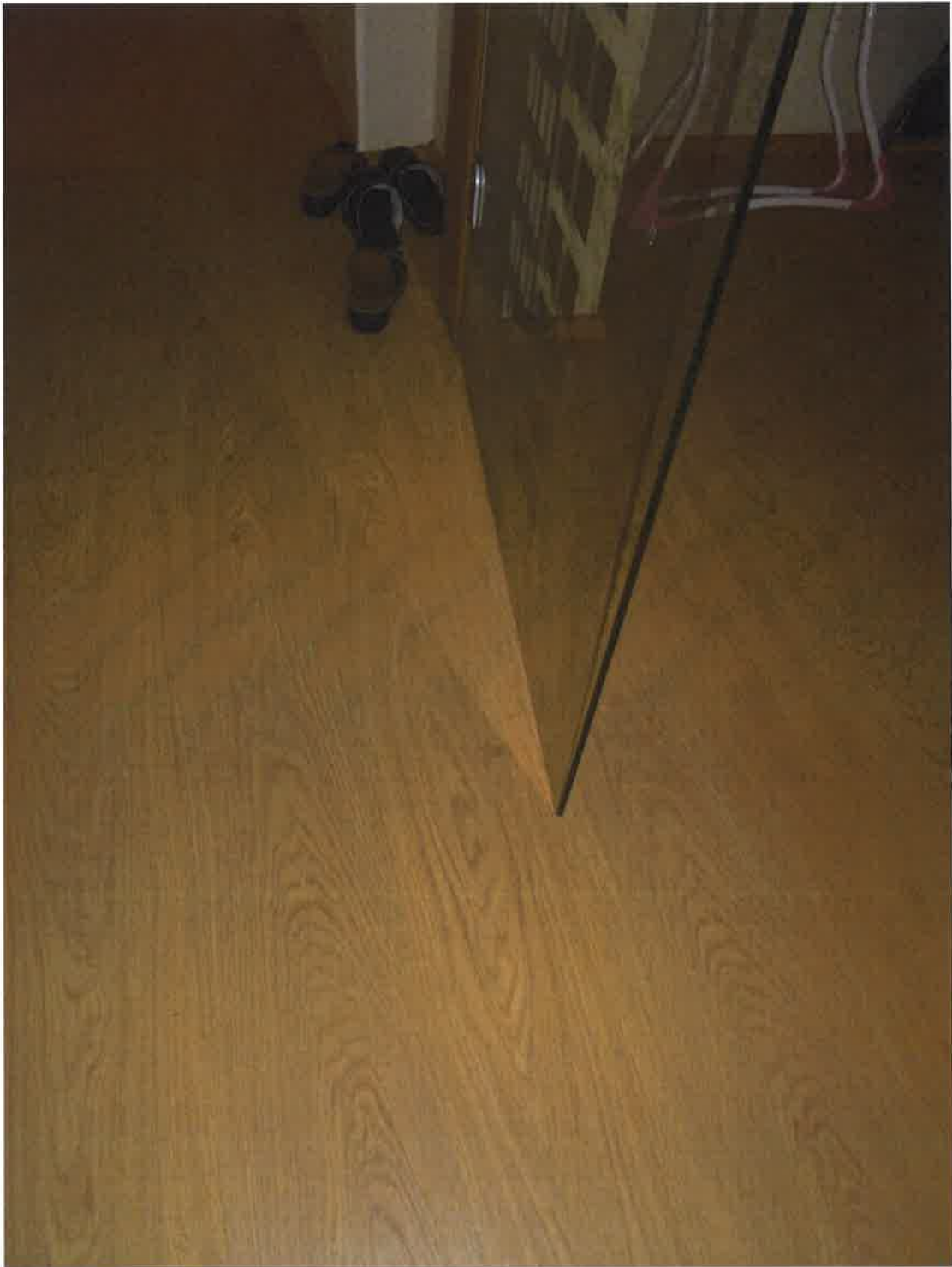
Lounge door sticking on floor
