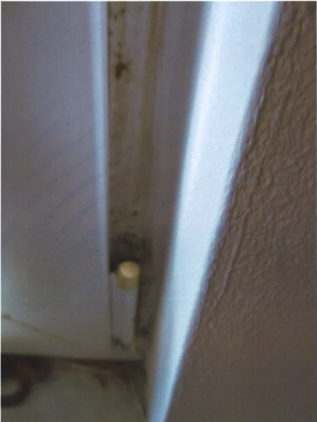
Mould around bedroom window 2
