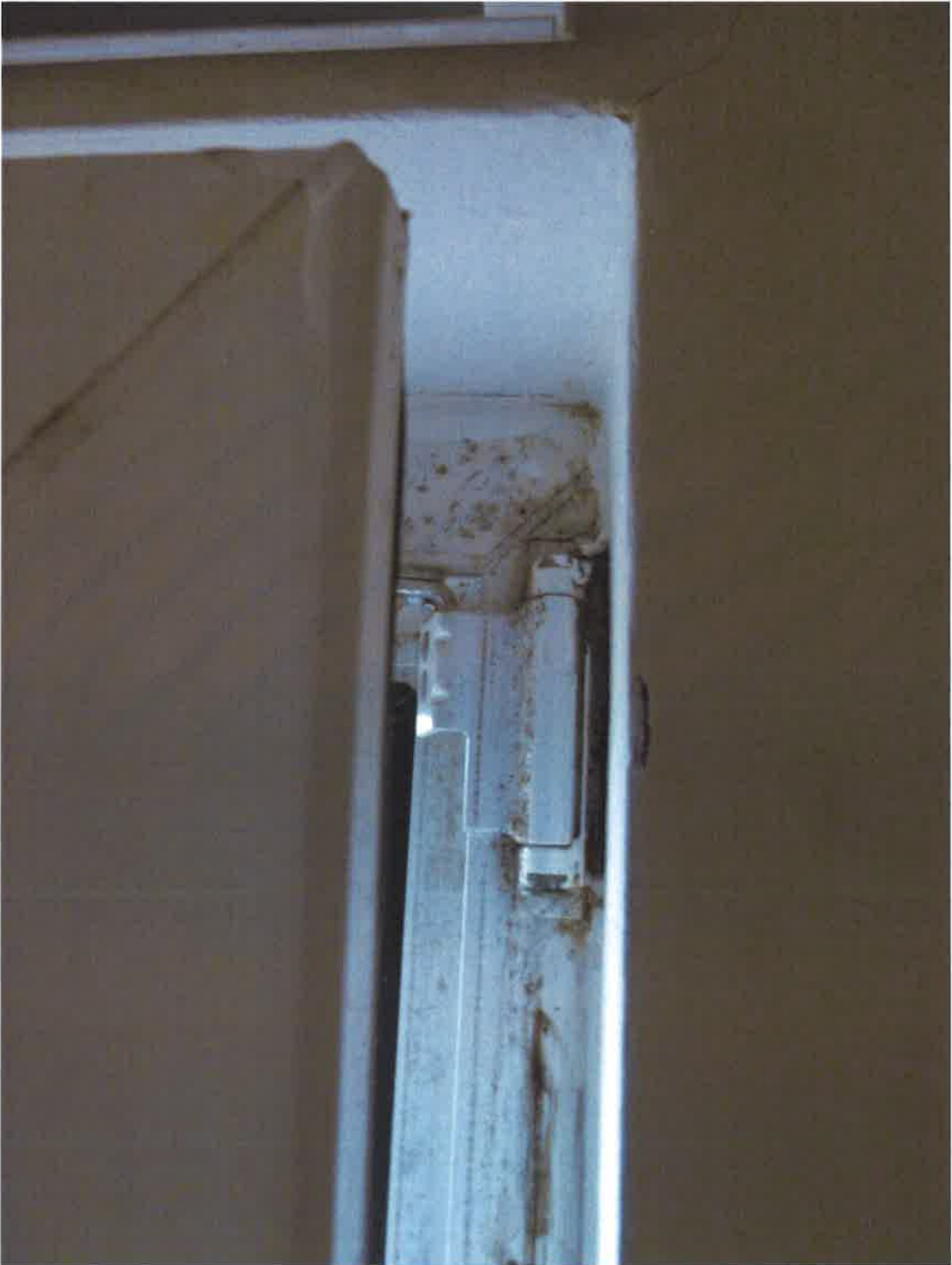
Mould around bedroom window 1
