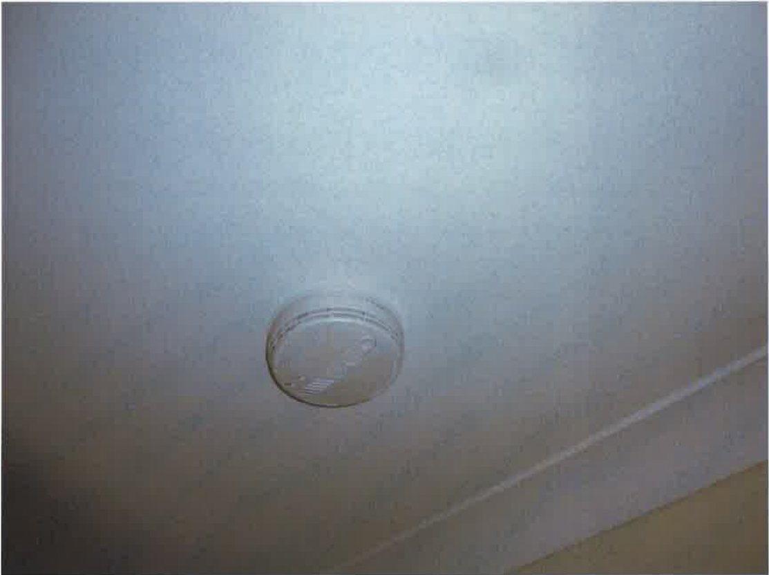
Upstairs smoke alarm
