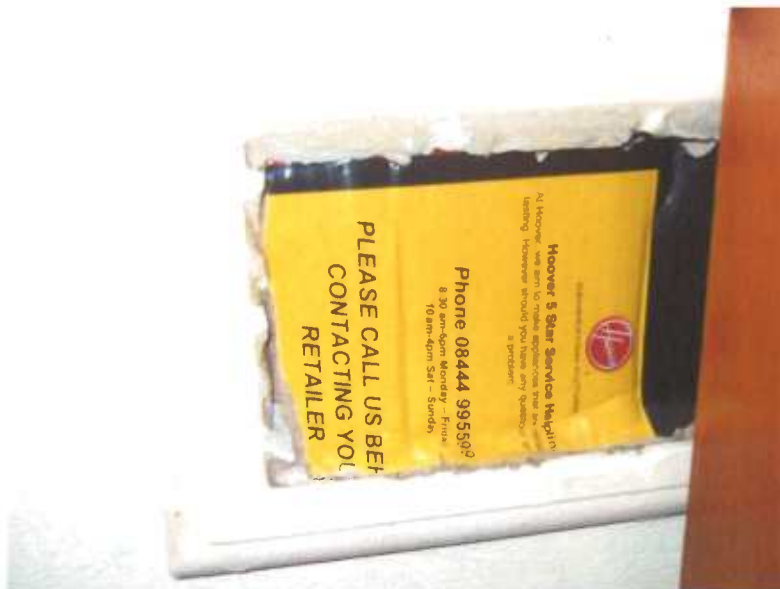
Missing vent cover – Rear right bedroom
