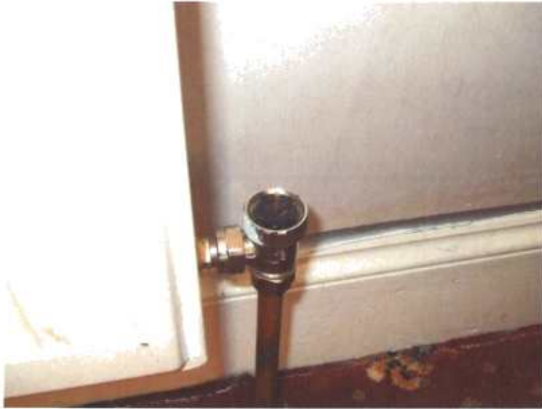
Defective radiator valve – one of several
