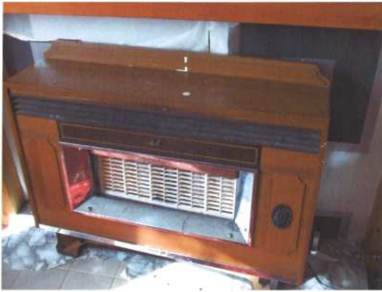
Disconnected gas fire – living room
