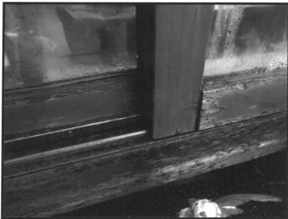
Figure 4 Patio door open joint
