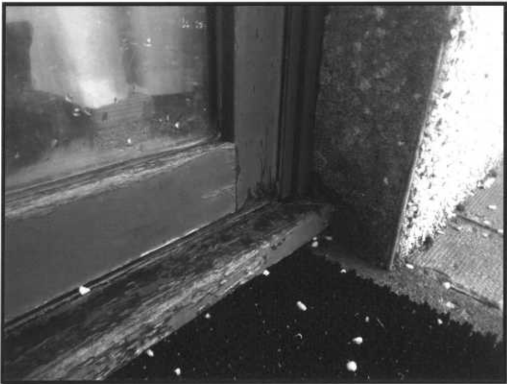
Figure 3 Decay to patio door
