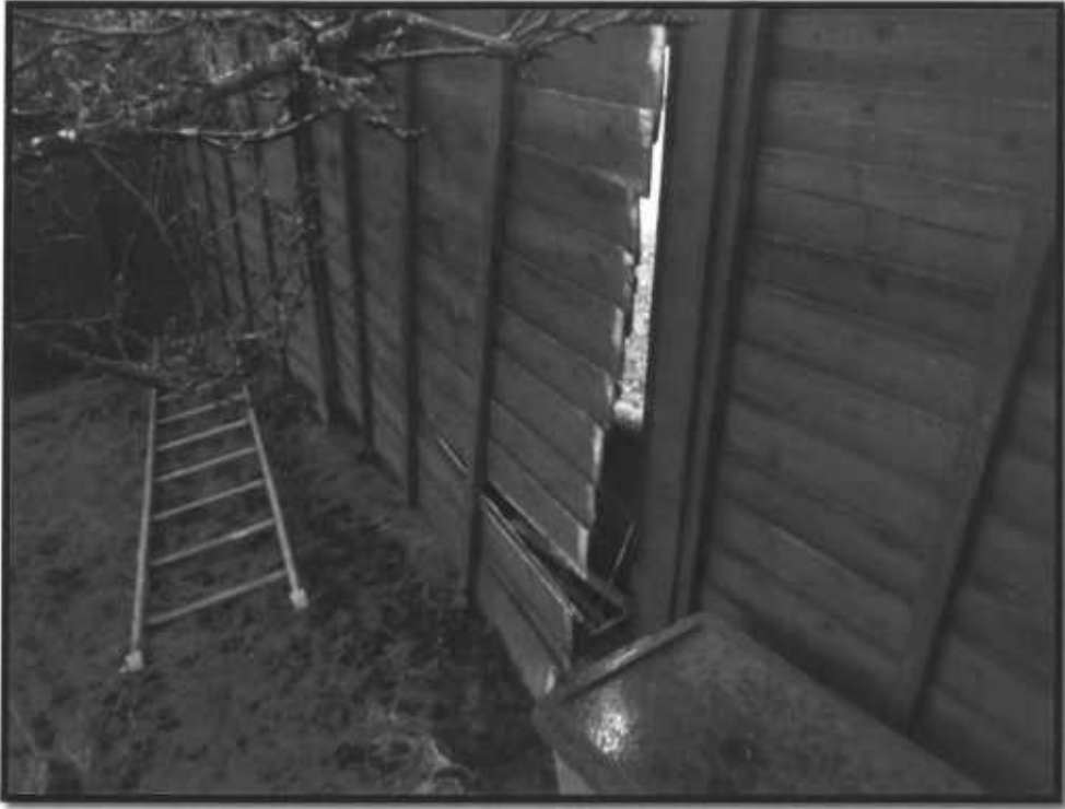
Figure 8 Example of damaged fencing
