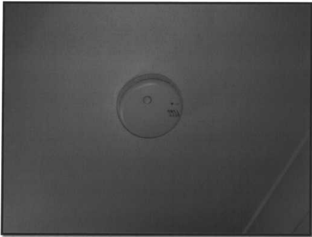
Figure 6 One of the hard wired smoke alarm
