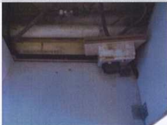
Wiring and socket in cabinet adjoining cooker hob
