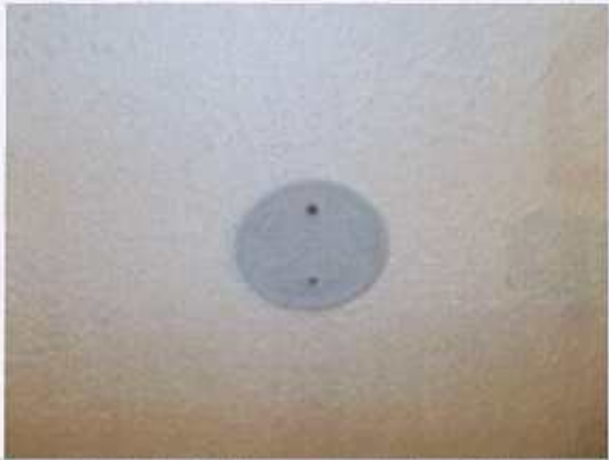
Smoke alarm fitting - GF Hall ceiling
