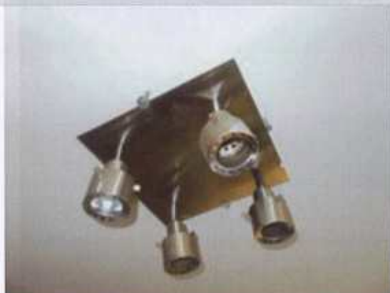
Light fitting to Kitchen ceiling
