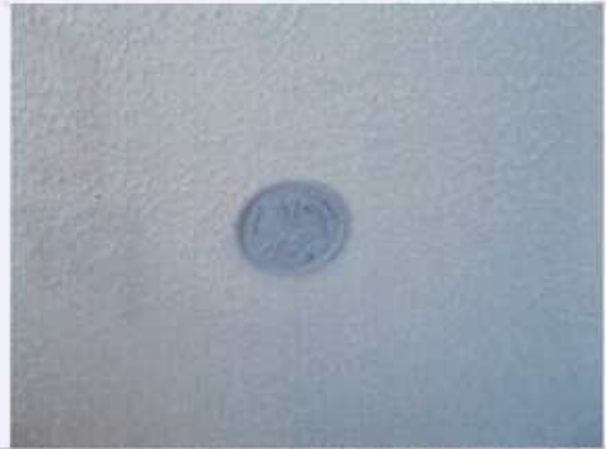
Smoke alarm fitting - UF Landing ceiling
