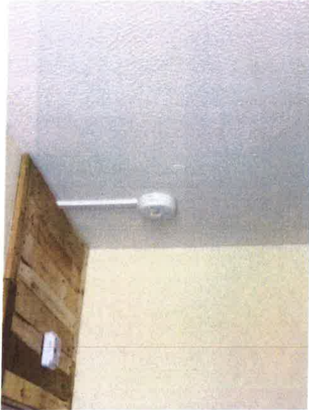
Heat detector – kitchen
