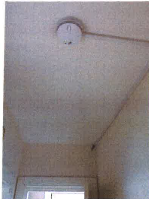
Smoke detector – hallway
