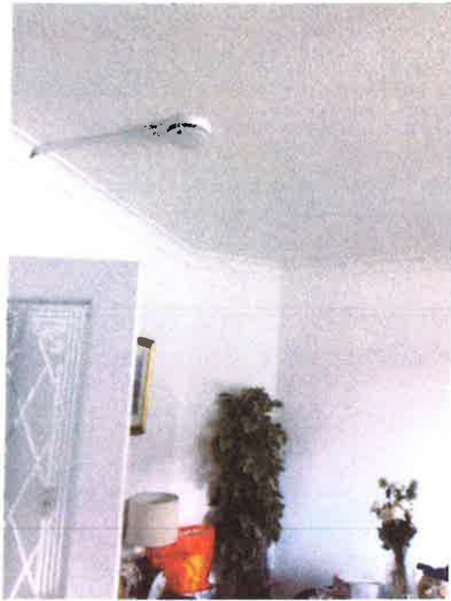
Smoke detector – living room
